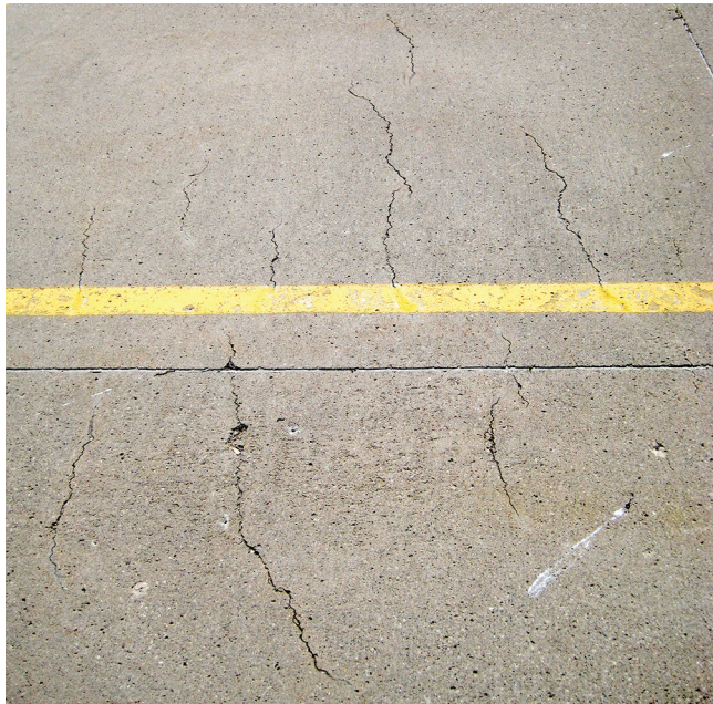
Figure 6-26. Plastic shrinkage cracks
