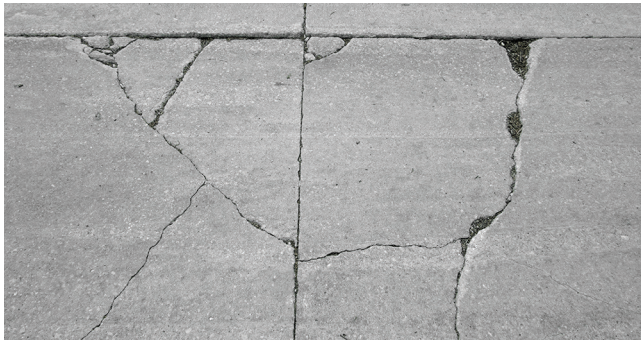
Figure 3-5. Corner cracking in jointed concrete pavement
