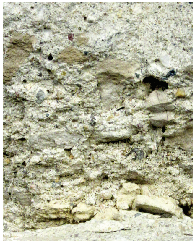
Figure 6-33. Joint damage showing flakes
