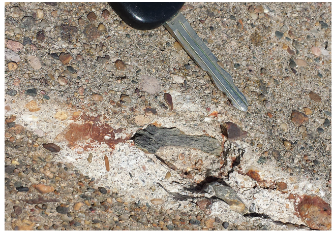
Figure 4-14. Popout at the concrete surface
