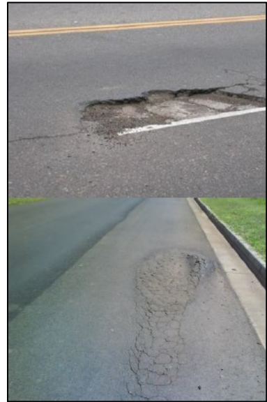
Damages to the flexible pavements due to weak geomaterial and soil characterizations
