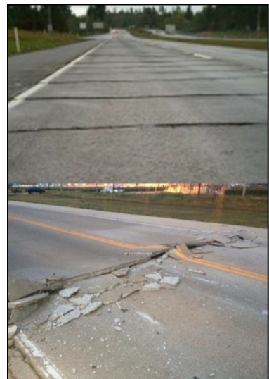
Damages to the rigid pavements due to weak geomaterial and soil characterizations
