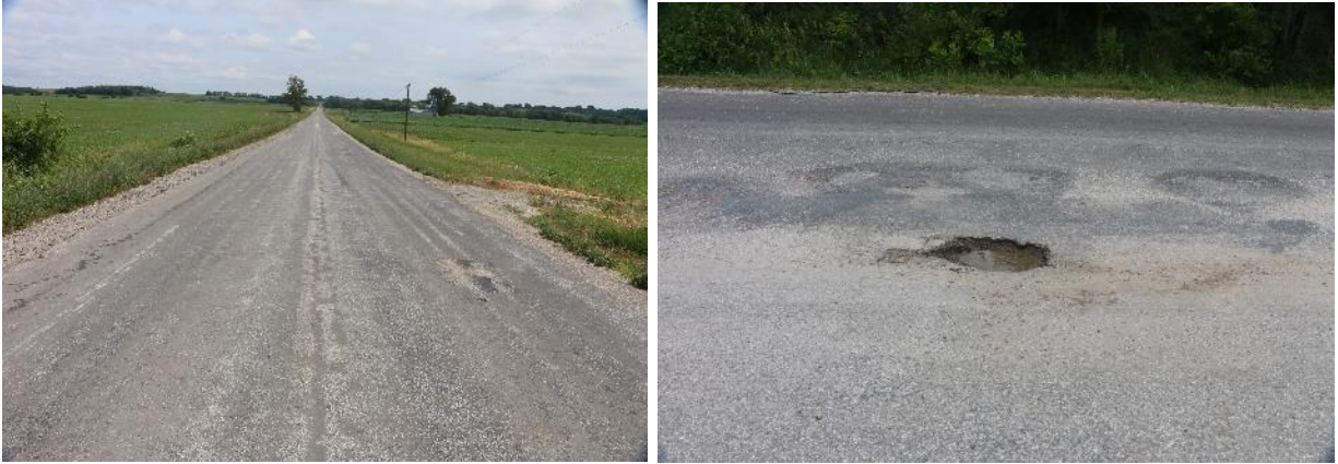
Figure 31. Condition of County Road J55 in Page County, Iowa, before implementing Otta seal (August 2020)
