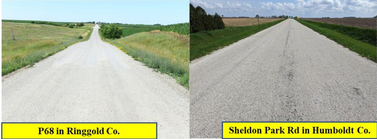
Figure B4. Otta seal site appearance in Ringgold County (photo taken on June 29, 2023) and Humboldt County (photo taken on May 12, 2023)
