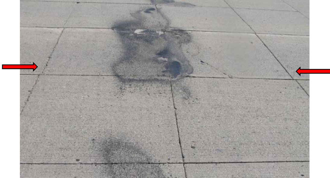
Figure 40 – Interior panels moving towards each other and blowup.
