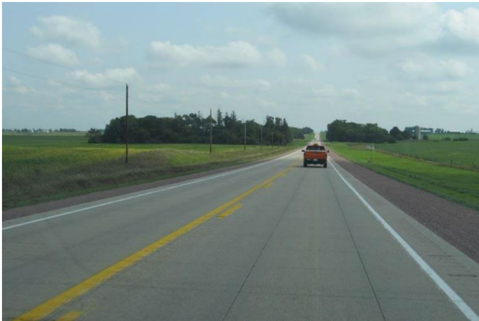
PCC overlay in better condition east of US 59.
