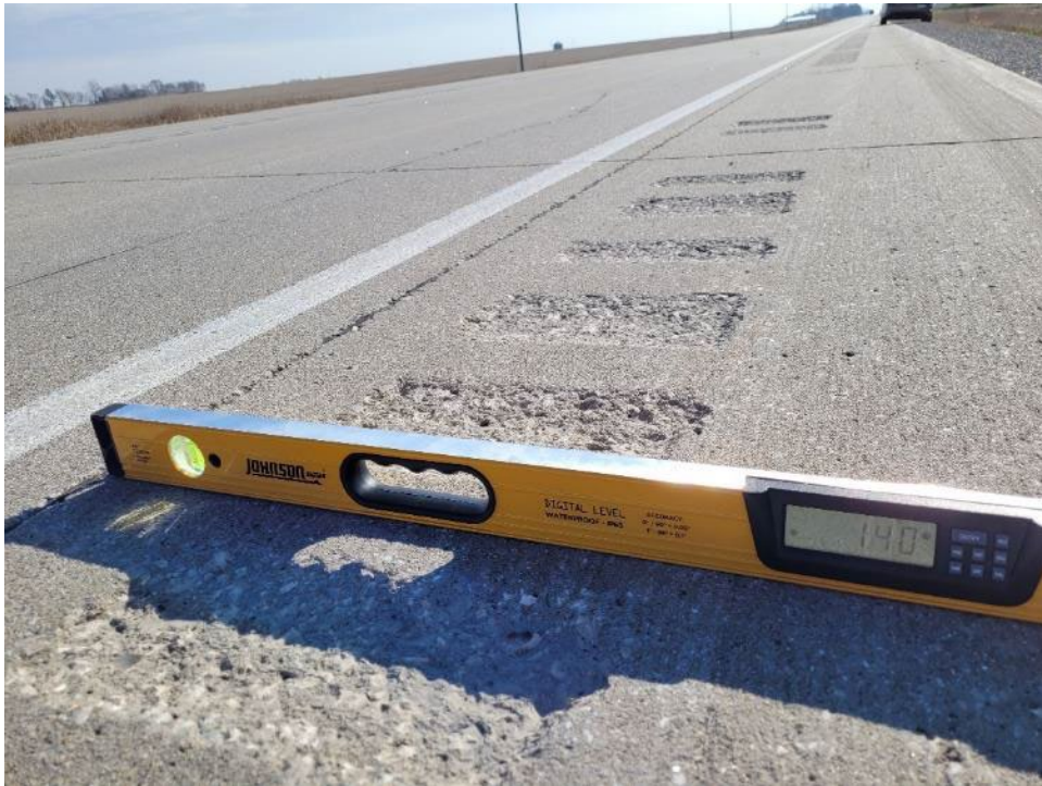
Figure 23 – Dallas US 169 UBOL Shoulder Cross Slope 1.40%
