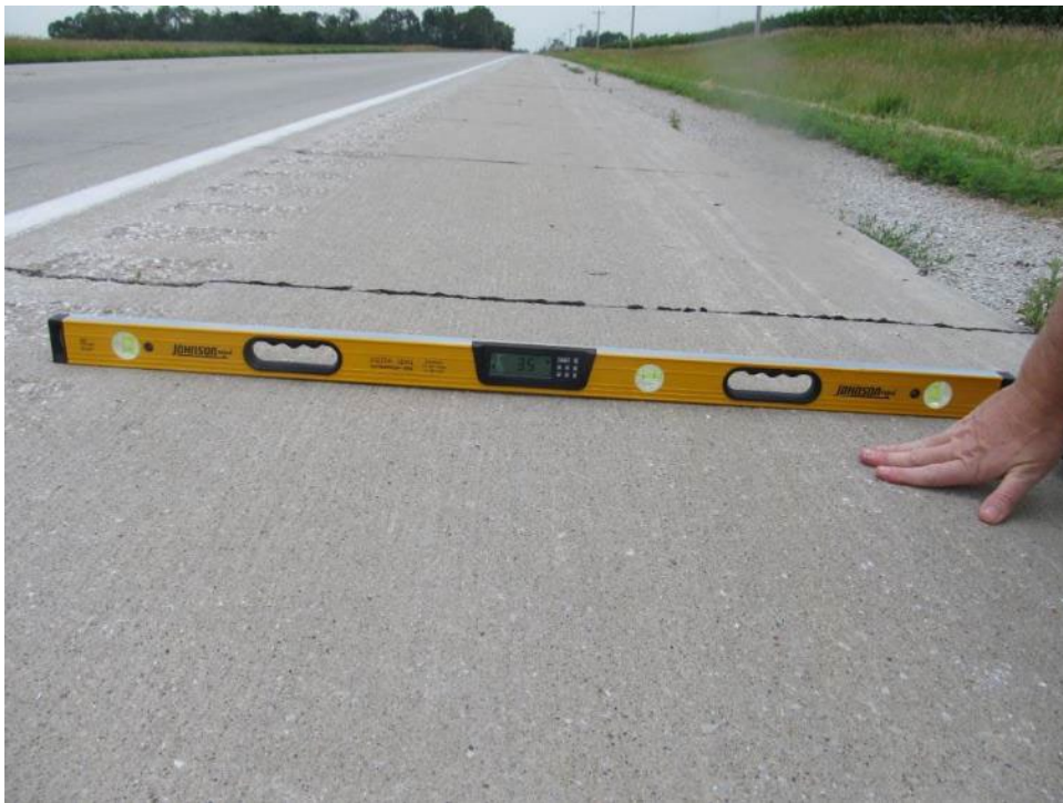
Shoulder cross slope 3.5%, Design 4%
