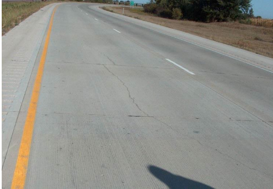
Figure 49 – Woodbury I-29 NB Longitudinal Cracking – passing lanes.
