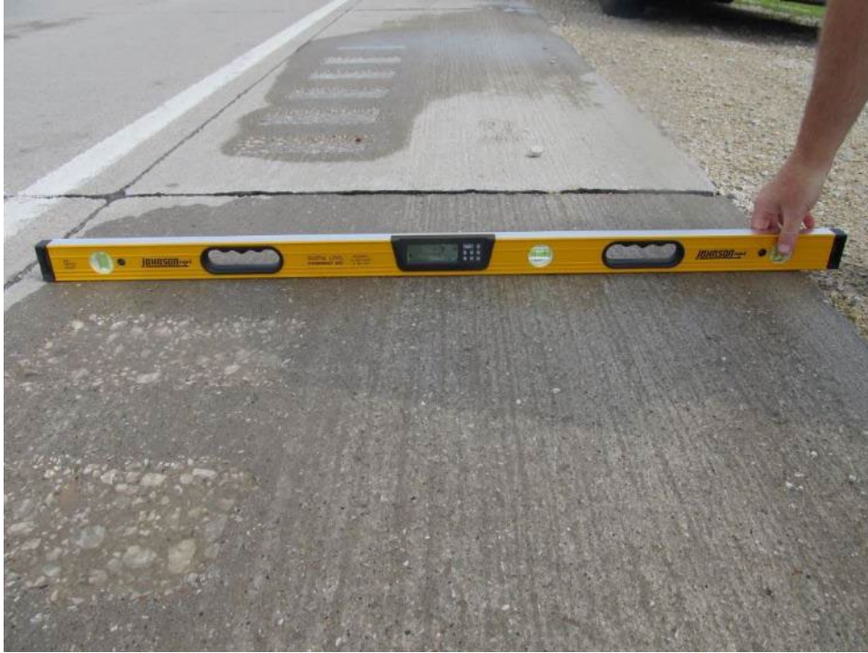
Shoulder cross slope 1.2%, Design 2%.
