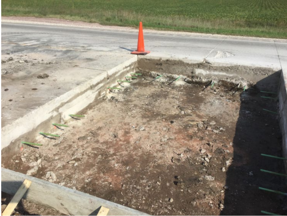
Figure 51 – Full depth PCC patch in overlay
