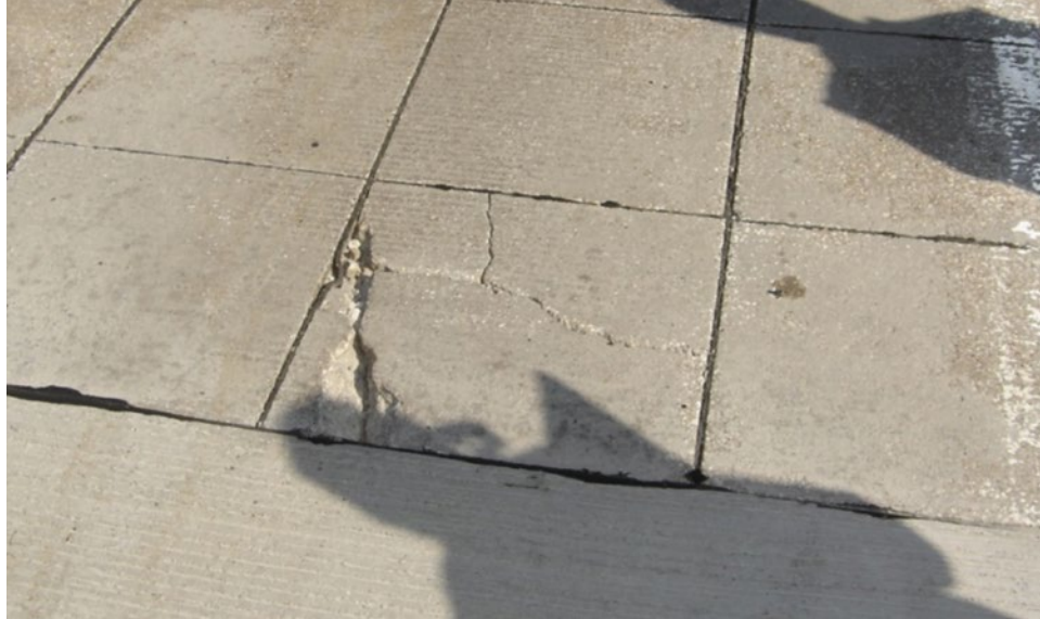
Figure 50 – Shattered panel. Typically overlay is thin in these areas.
