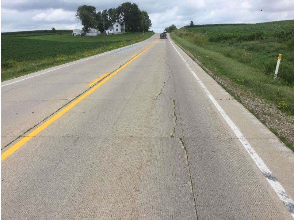
Figure 9 – Delaware IA 13 Widening Unit Heaving
