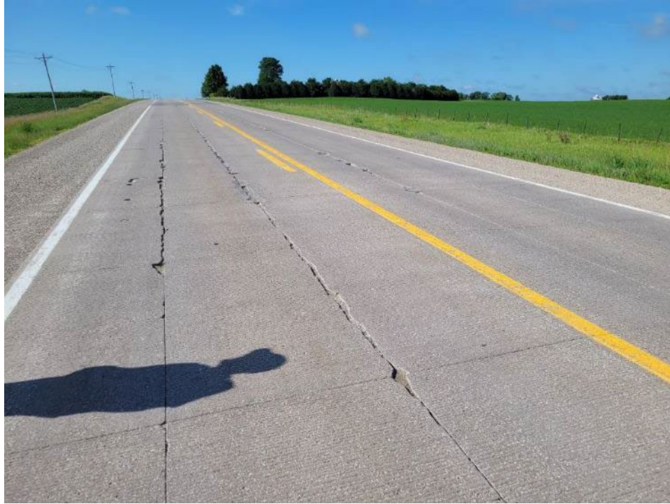
Figure 7 – 4-inch Overlay 4 x 4 ft. Joint Spacing exhibiting some joint deterioration.
