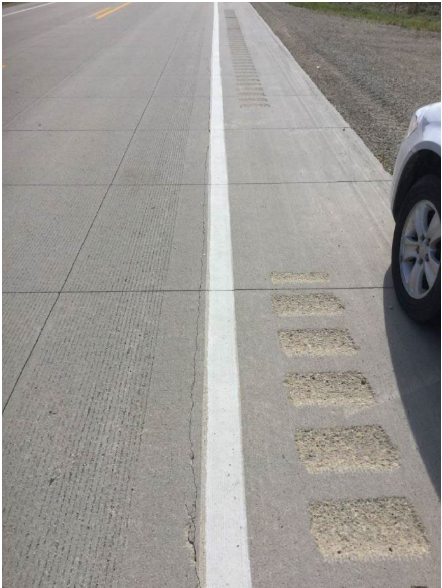
2017 – Cracking at 4 ft from edge. Location of old edge of widened pavement.
