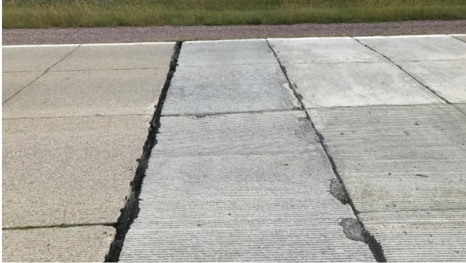
Figure 53 – Panel placed with 1 inch gap. Do NOT leave space.
