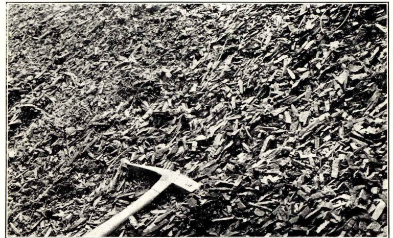
Fig. 8. Detail of weathering of shale, near Norton, Virginia. Taken with auxiliary lens of portrait type. Example of satisfactory definition wrought over oblique field with a very imperfect optical system by means of very small aperture.
