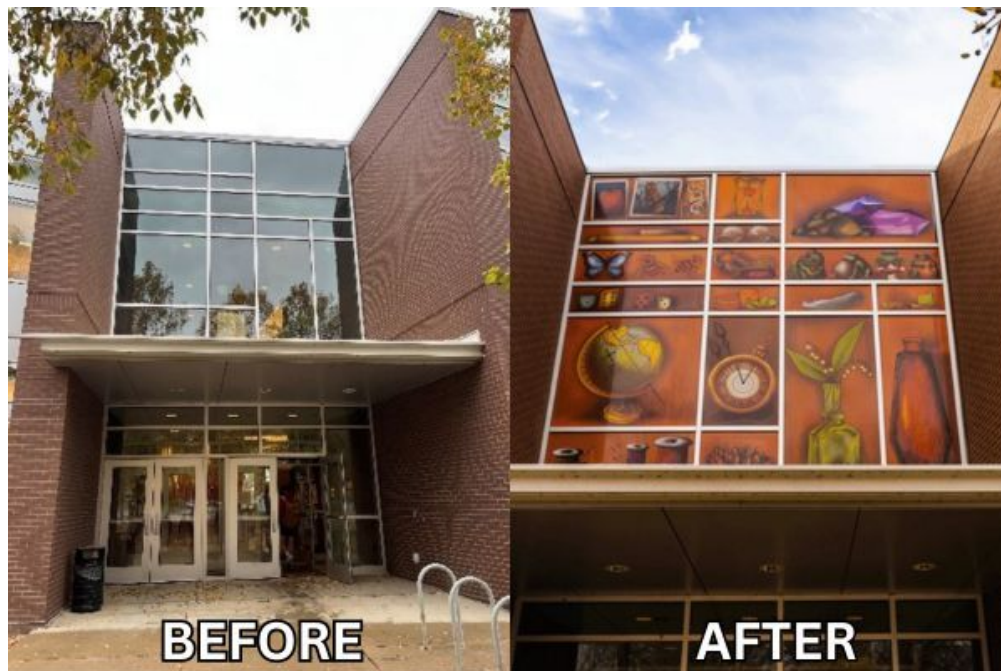
The Roe Center at Central College, before and after decals were installed to reduce bird collisions with windows.
