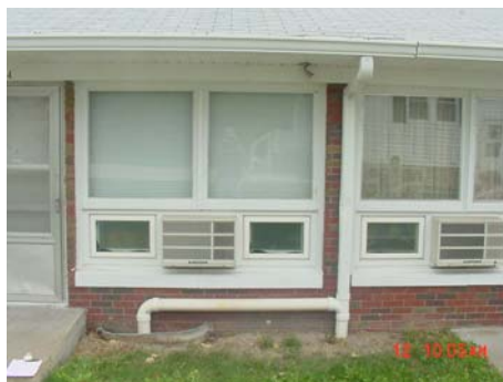
This is the continuation of the dryer vent and where it hooks into the gutter system.
