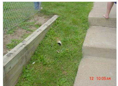
Does the exhaust go up the downspout, or could this be where the exhaust terminates? Maybe a little bit of both? A renter indicated the exhaust terminates here. Wow!
