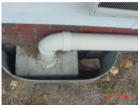
Above is a plywood box where two dryer terminations dump their exhaust.
