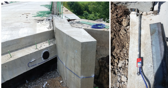
Earth pressure sensor on abutment backwall (left) and crackmeter on approach slab surface (right)
