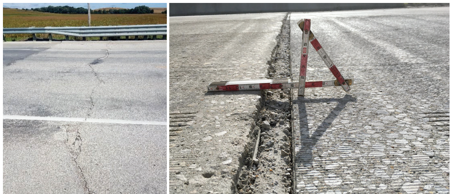
Transverse cracking in approach slab (left) and differential settlement at joint (right)
