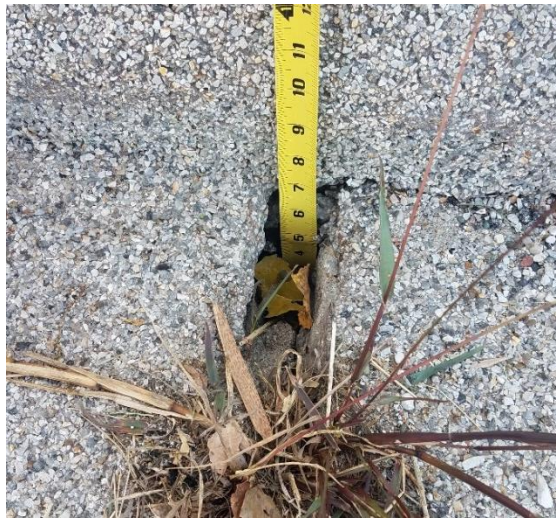
Figure 3.4. Void at the intersection of bridge-deck-to-approach-slab joint and barrier
