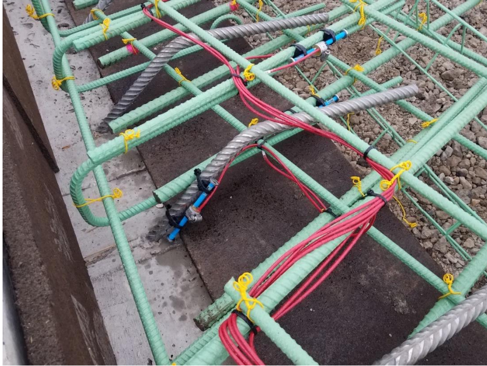
Figure 4.26. Story County 118—strain gauges installed on the longitudinal rebar and tie bars
