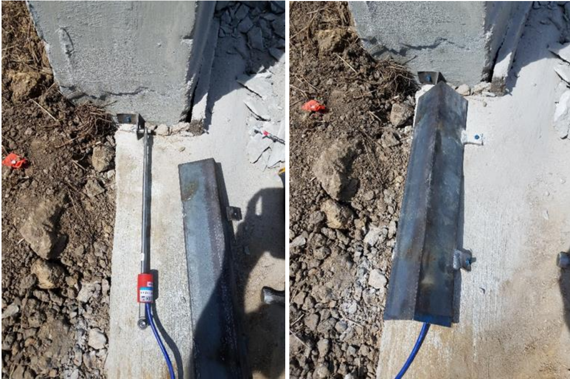
Figure 4.6. Jasper County 118—crackmeter without protective cover (left) and crackmeter with protective cover installed (right)
