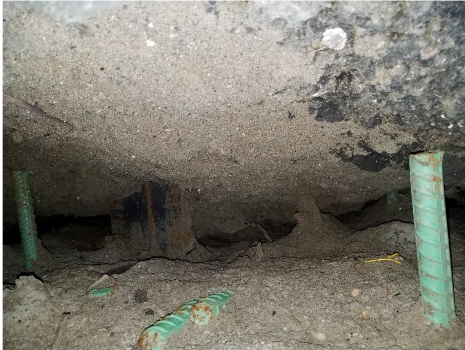
Figure 4.45. Story County 118—visible exposed rebar and foundation pile
