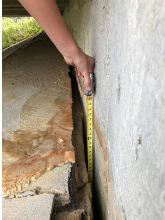
Figure 3.13. Measuring tape showing the vertical depth of the void
