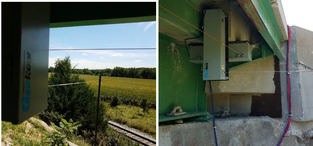
Figure 4.7. Jasper County 118—displacement transducer with reference post (left) and longitudinal and transverse displacement transducers attached at the acute bridge corner (right)
