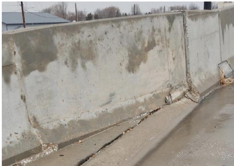
Figure 2.34. Cracking at barrier
