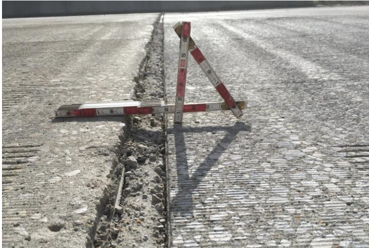
Figure 2.29. Differential settlement at joint
