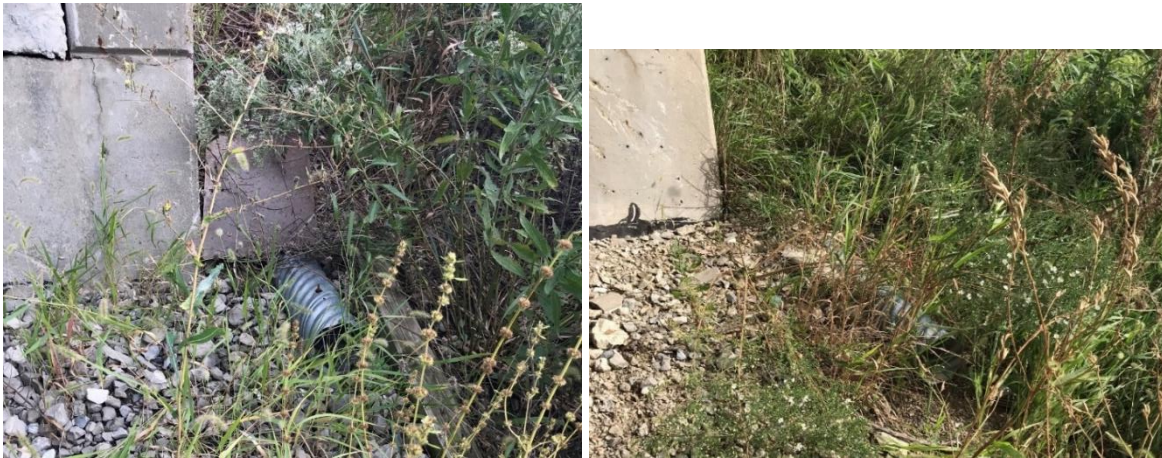
Figure 3.9. Blocked embankment drainage (left) and additional blocked embankment drainage (right)
