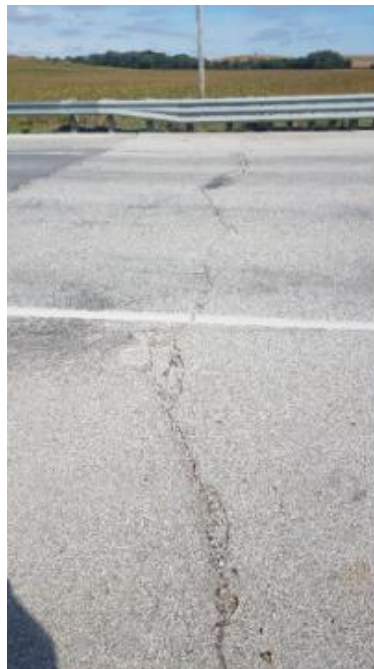
Figure 2.26. Transverse cracking of approach
