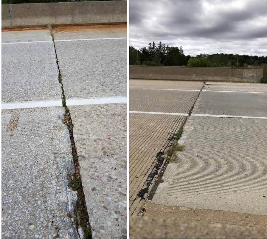
Figure 3.10. Deck-to-approach-slab joint showing severe spalling (left) and additional deck-to-approach-slab joint showing severe spalling (right)
