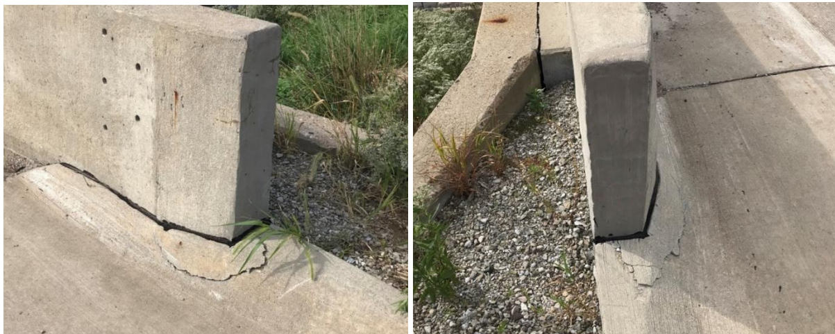
Figure 3.8. Concrete cracking at the end of the wingwall (left) and additional cracking at the end of the wingwall (right)
