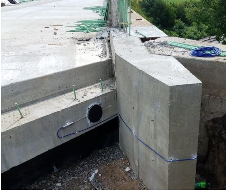
Figure 4.4. Jasper County 118—EP1-W earth pressure sensor after installation
