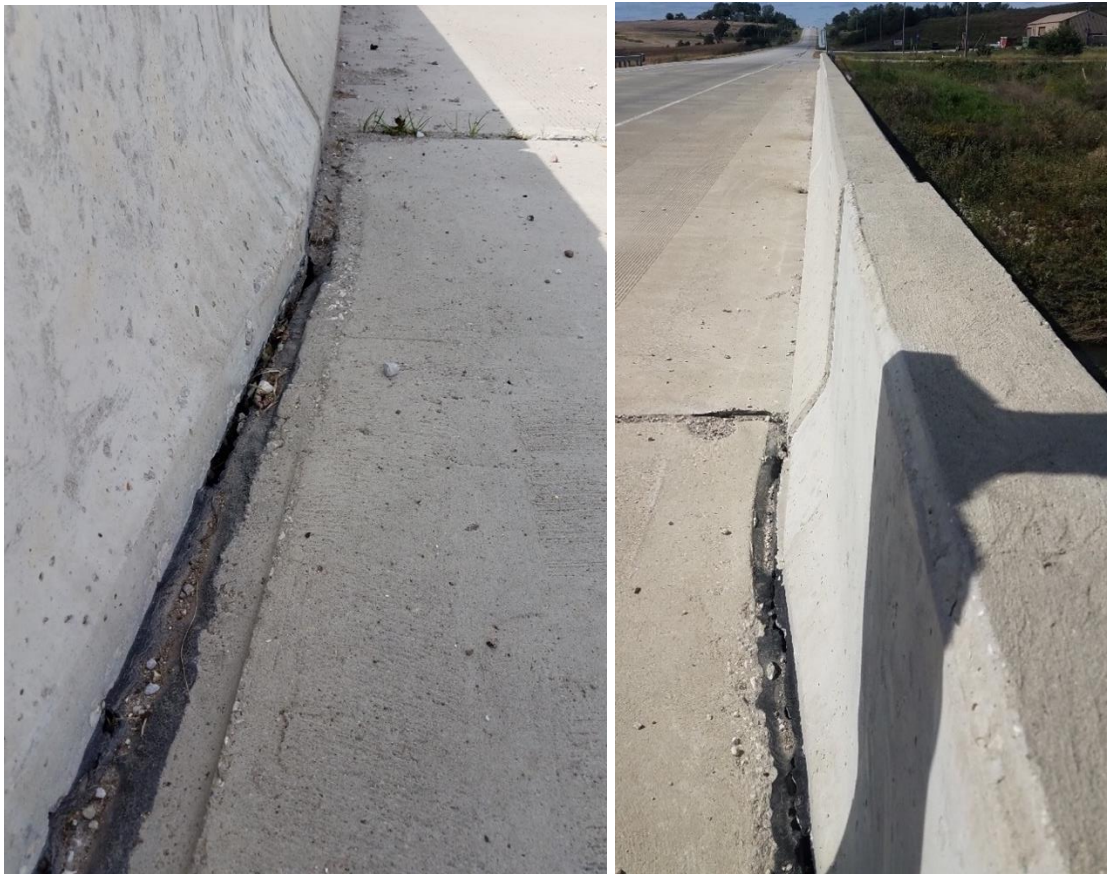
Figure 3.5. Approach-slab-to-wingwall joint showing separation (left) and misaligned wingwall and barrier (right)
