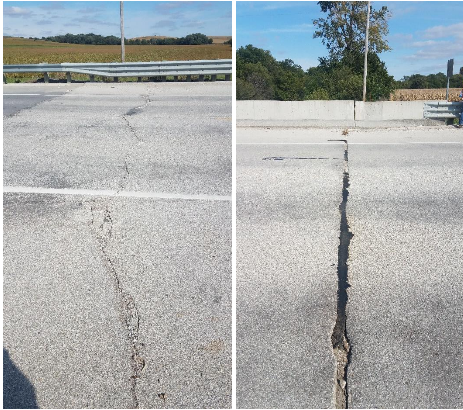
Figure 3.3. Transverse approach slab crack (left) and bridge-deck-to-approach-slab joint (right)
