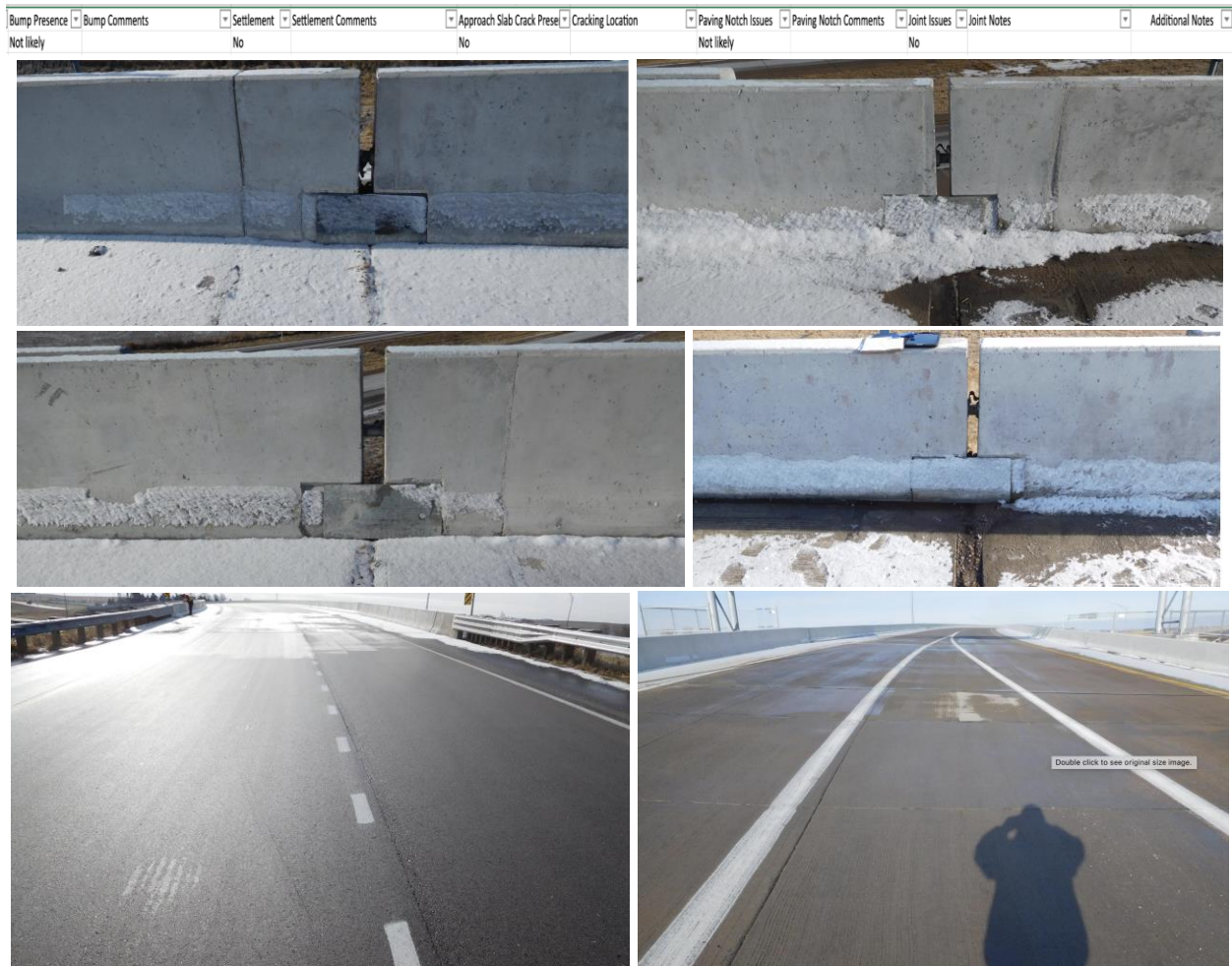
Figure 2.49. Bridge issues table and bridge inspection photographs
