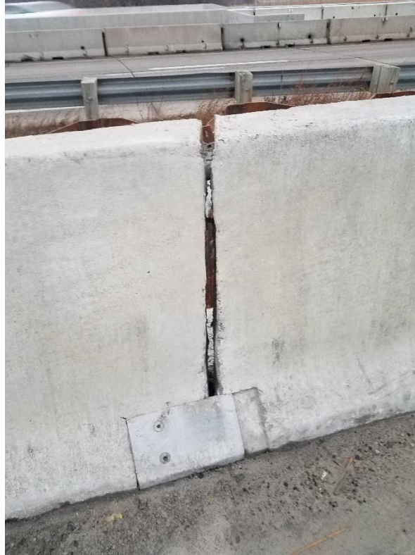
Figure 4.41. Story County 118—open barrier joint (typical)
