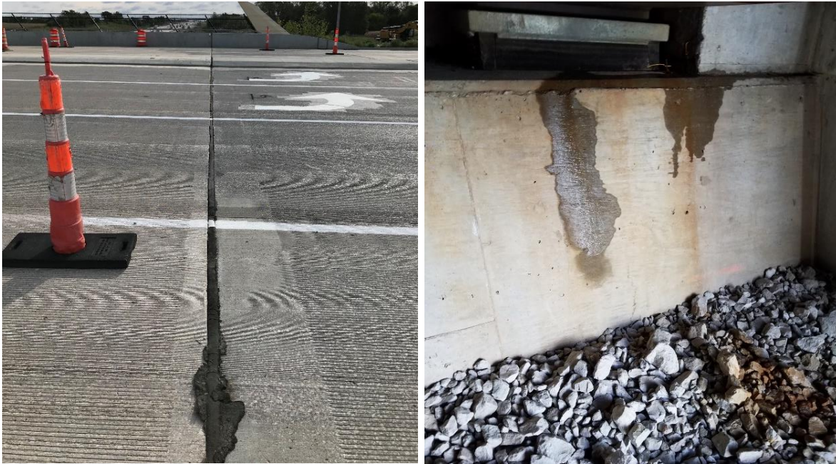
Figure 3.1. South bridge-deck-to-approach-slab joint with excess sealant (left) and water and abutment staining at the outermost girder (right)
