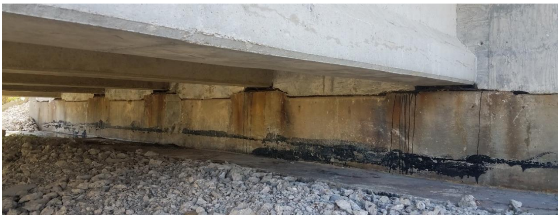
Figure 3.7. Abutment face showing the new backwall on top of the old footing
