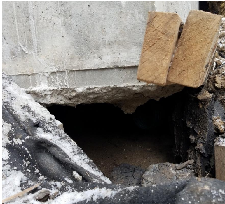
Figure 4.44. Story County 118—large void under the south abutment corner
