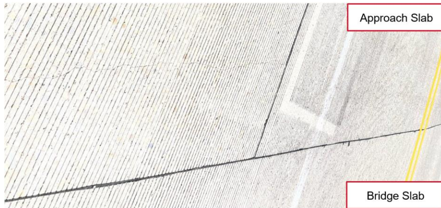
Figure 4.73. Butler County 118—transverse crack on the east approach slab
