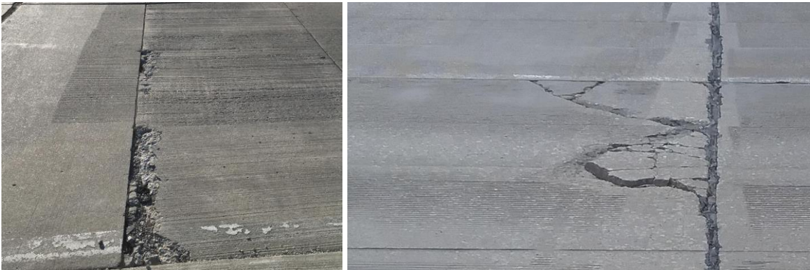
Figure 2.30. Examples of spalling
