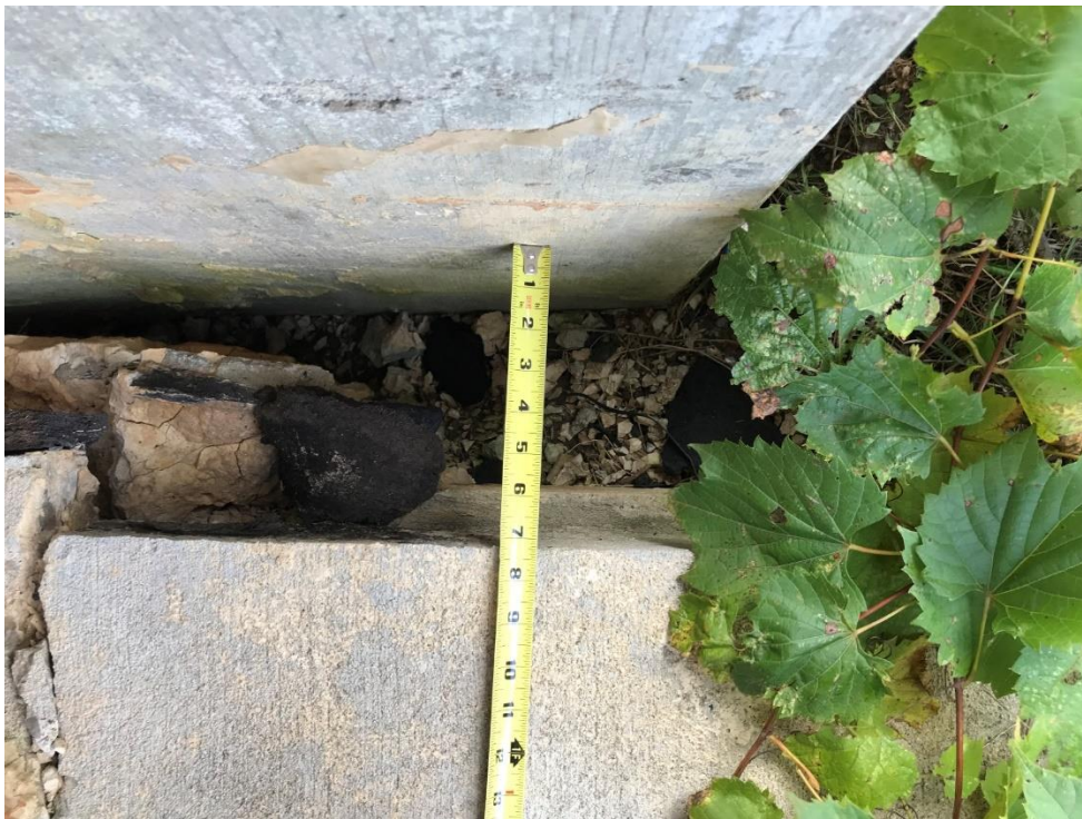
Figure 3.12. Horizontal void created by the embankment pulling away from the abutment
