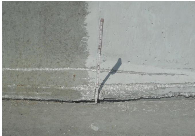
Figure 2.28. Differential settlement at barrier
