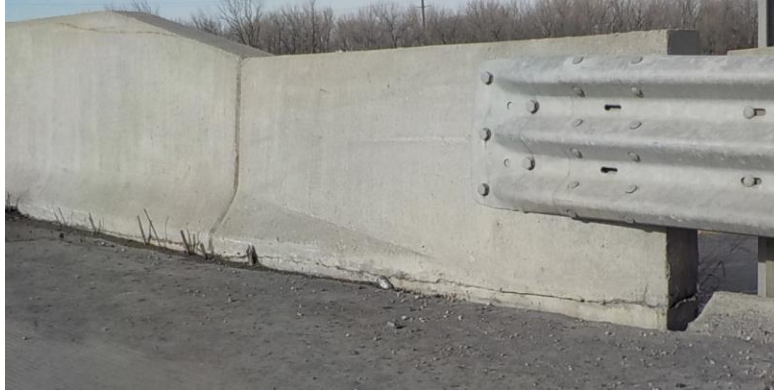
Figure 2.33. Cracking/Differential settlement at barrier
