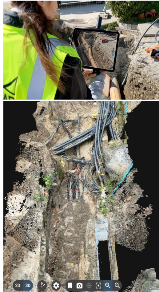
Figure 7. Pix4D is easy to deploy and readily provides spatially accurate, high resolution digital as-built positional and geometric data of open trench and surface utility installations.
