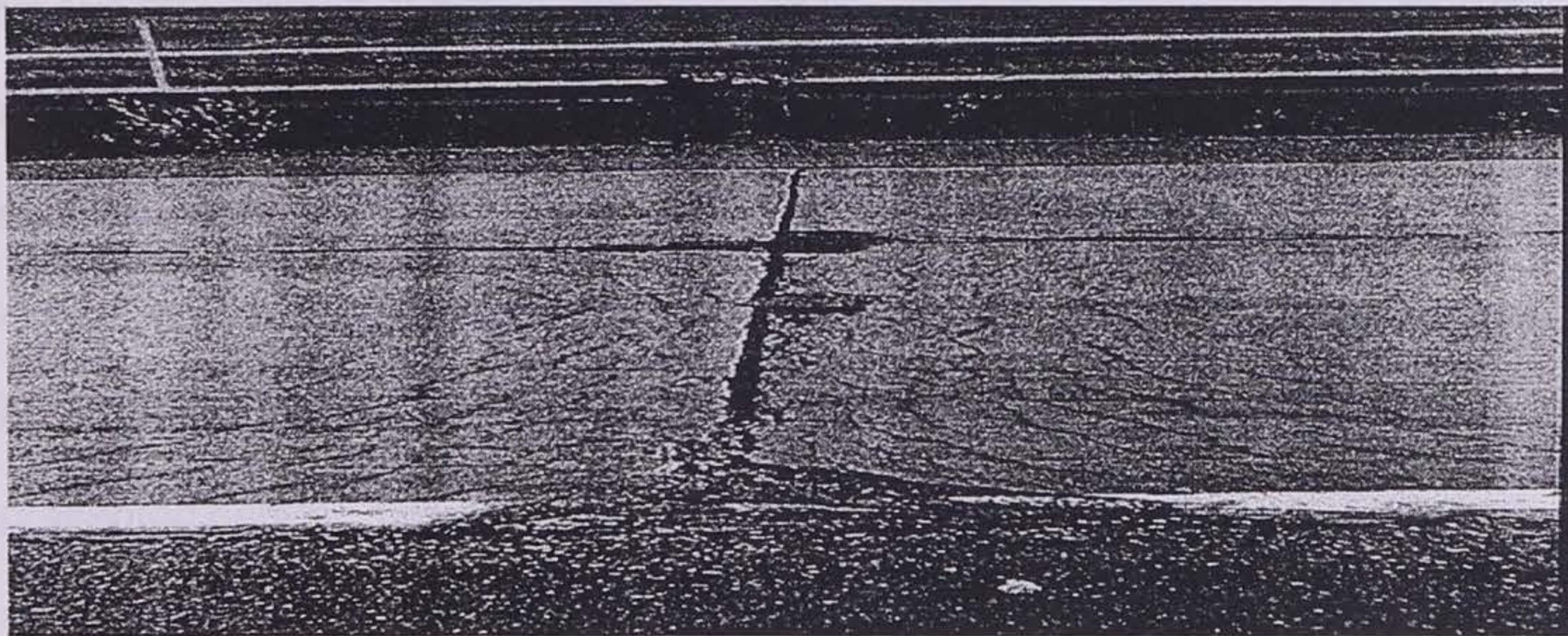
Figure 1 Transverse Joint Failure in Concrete Pavement
