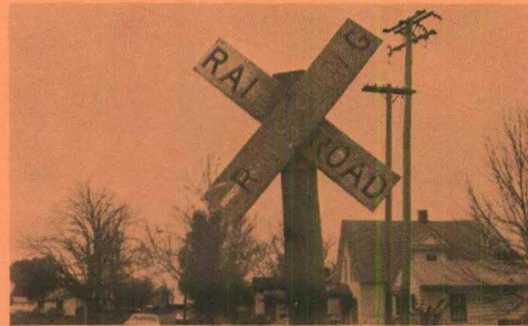
E-2 SW WALNUT STREET--Deteriorated Crossbuck
