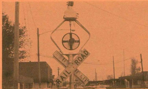
G-2 SW 3rd STREET--Deficient Maintenance Of Substandard Equipment
