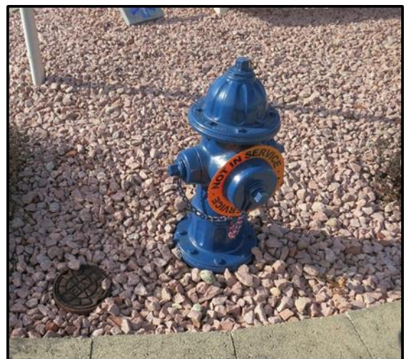
New hydrant, not yet in service
