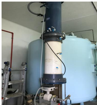
Pilot project for ammonia removal
