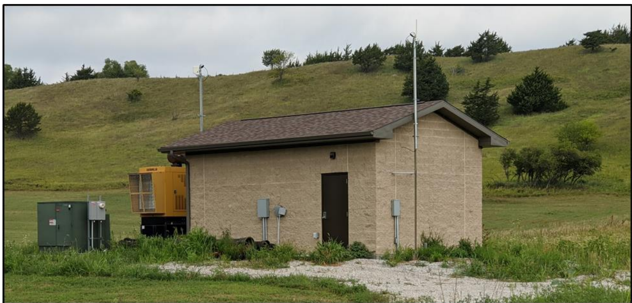
Well house with emergency generator
