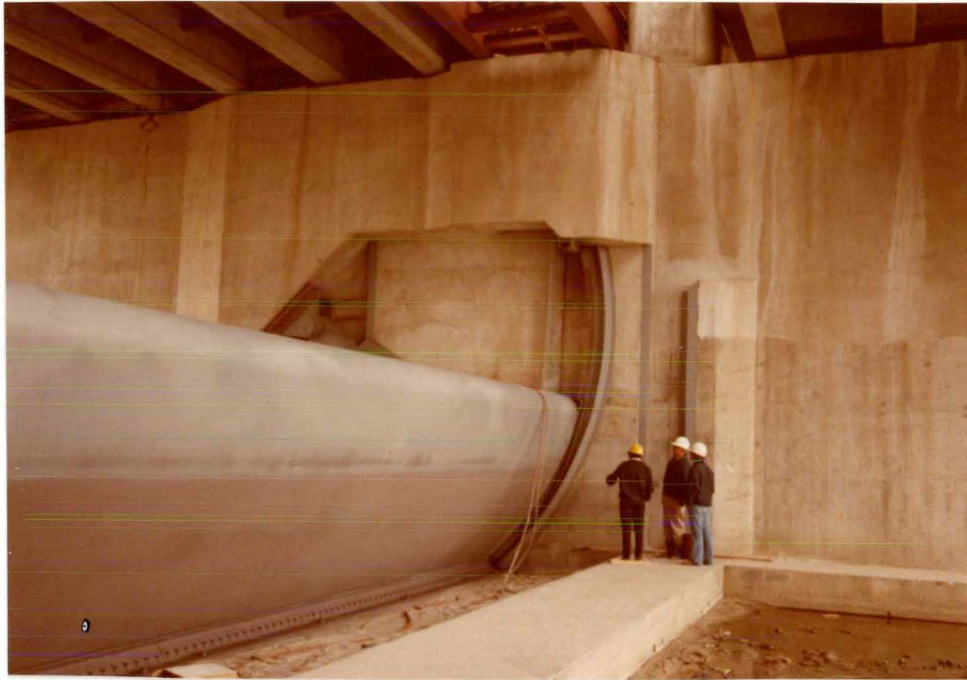
Upstream face of one of the four 85-ton submersible taintor gates. Each of these gates is 16 feet high, 6 feet thick, and 60 feet long.
