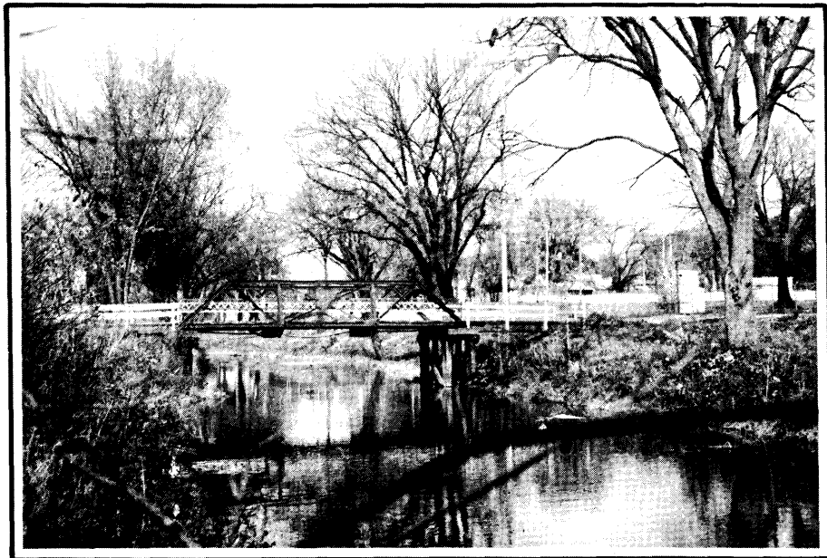
Thomas Park Bridge Mile 10.65. Looking Upstream at lower vehicular bridge within the City Park, swimming pool upstream on right bank.
