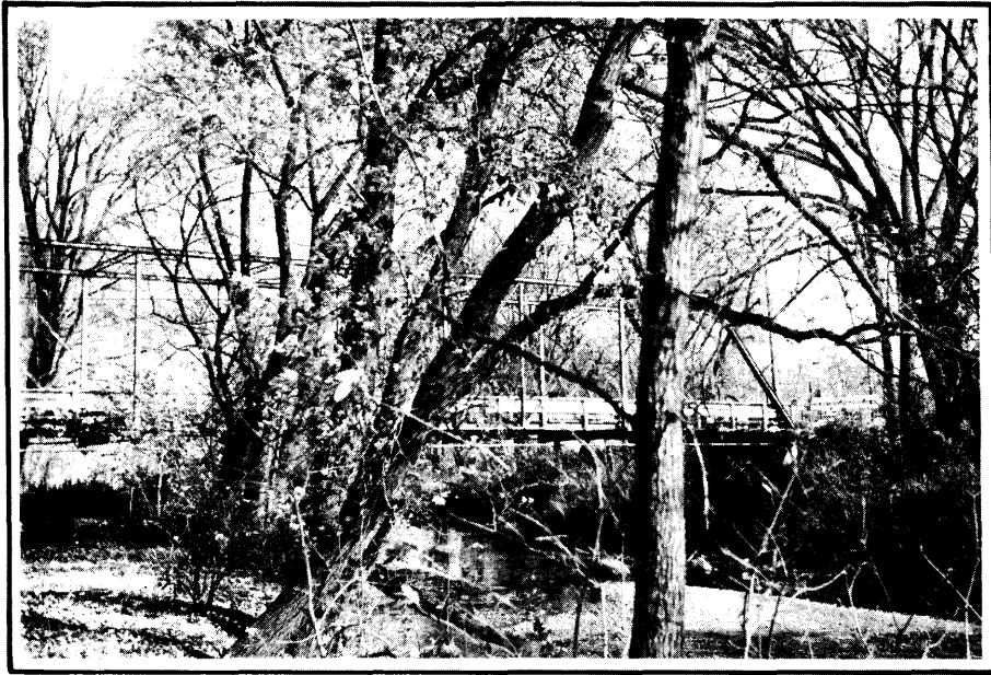
County Road "GG" Bridge Mile 0.75. Looking Upstream at Bridge with approach span on Right Bank on wood piling.
