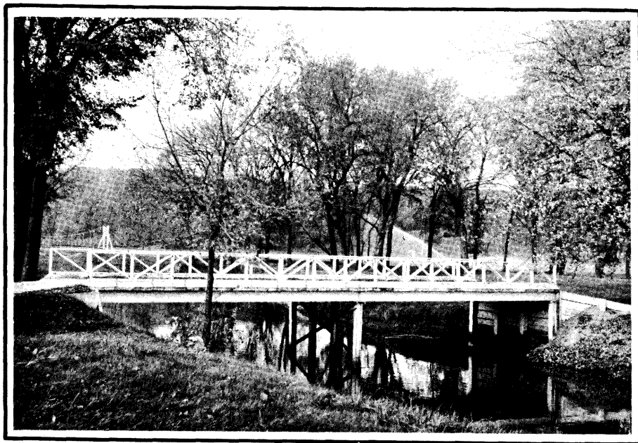
Cedar Rapids Country Club Maintenance Bridge Mile 5.80. Looking Downstream with suspension footbridge in background.
