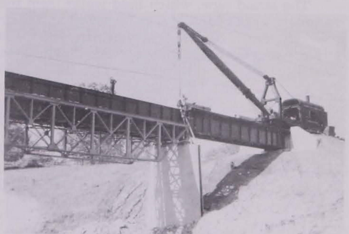
Constructing a new bridge on the Ainsworth to Brighton cutoff. 3 1/2 miles So. of Washington over crooked creek. May, 1947.
