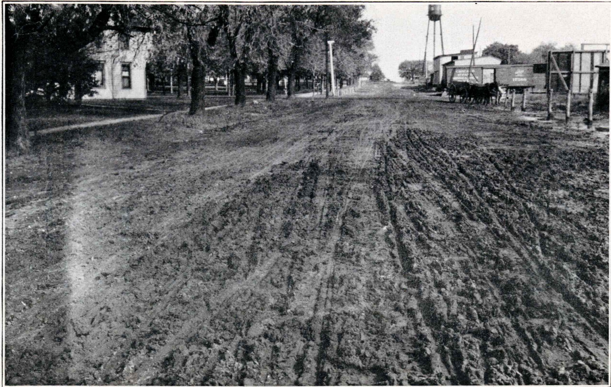
A street in Ames, Iowa, looking from the part not oiled onto the part that was oiled in July for the first time. Photographed in October after a week of wet weather.
