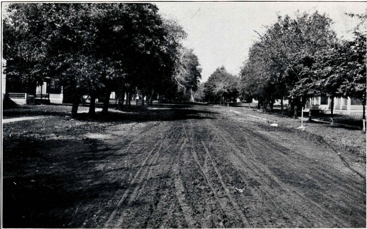
This is how an oiled street looks after several days of rain. Note that only a small amount of mud has resulted. This street is well rounded up, which is essential for proper drainage.
