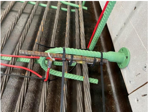
(c) Strain gauge at the bottom of a box girder
