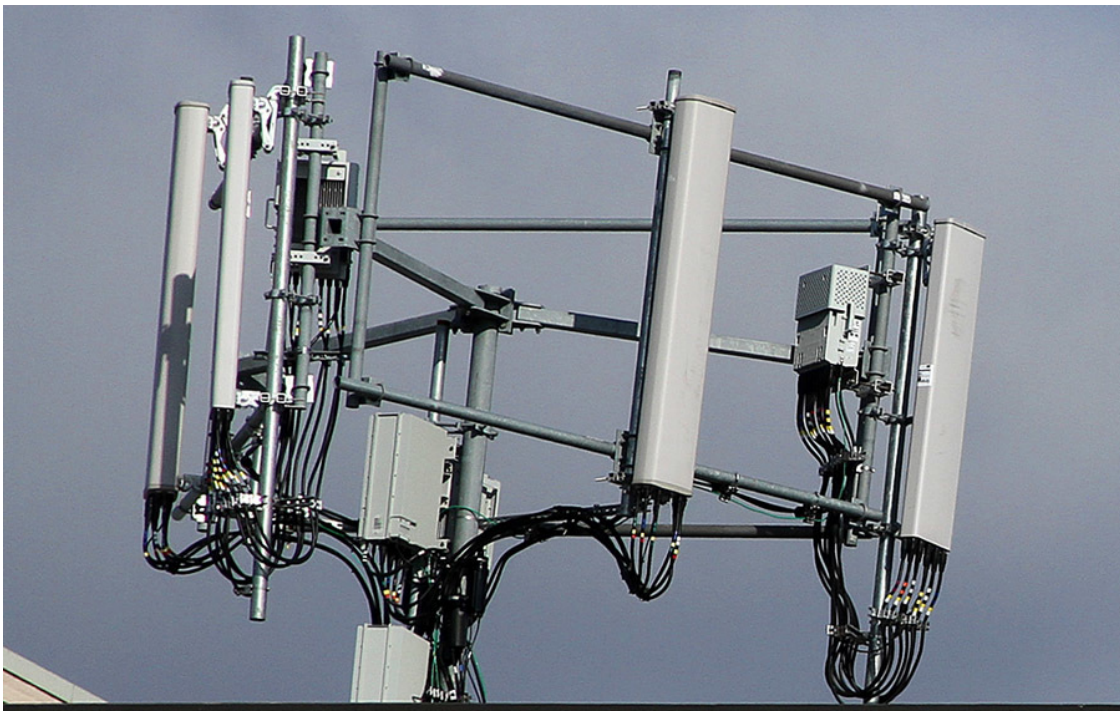
Des Moines rooftop cellular tower.
