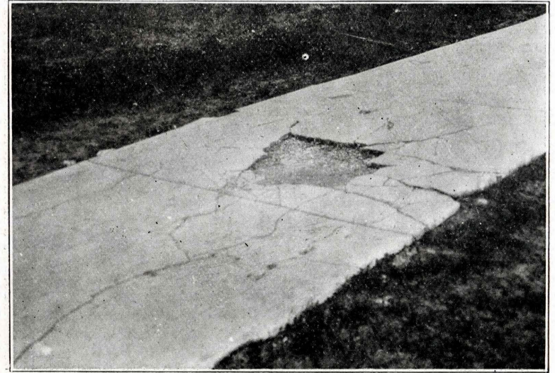
This walk appears to be of very poor concrete throughout.
