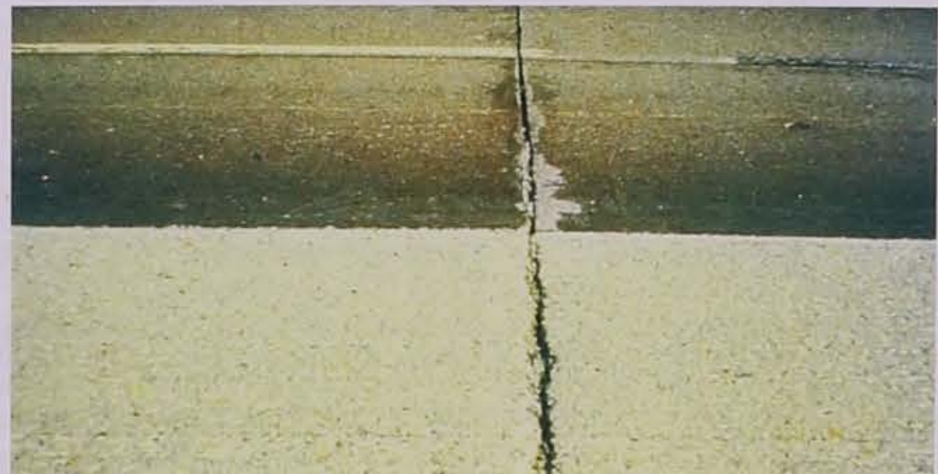
Figure 9.8. Joint damage (foreground) caused by cold milling
