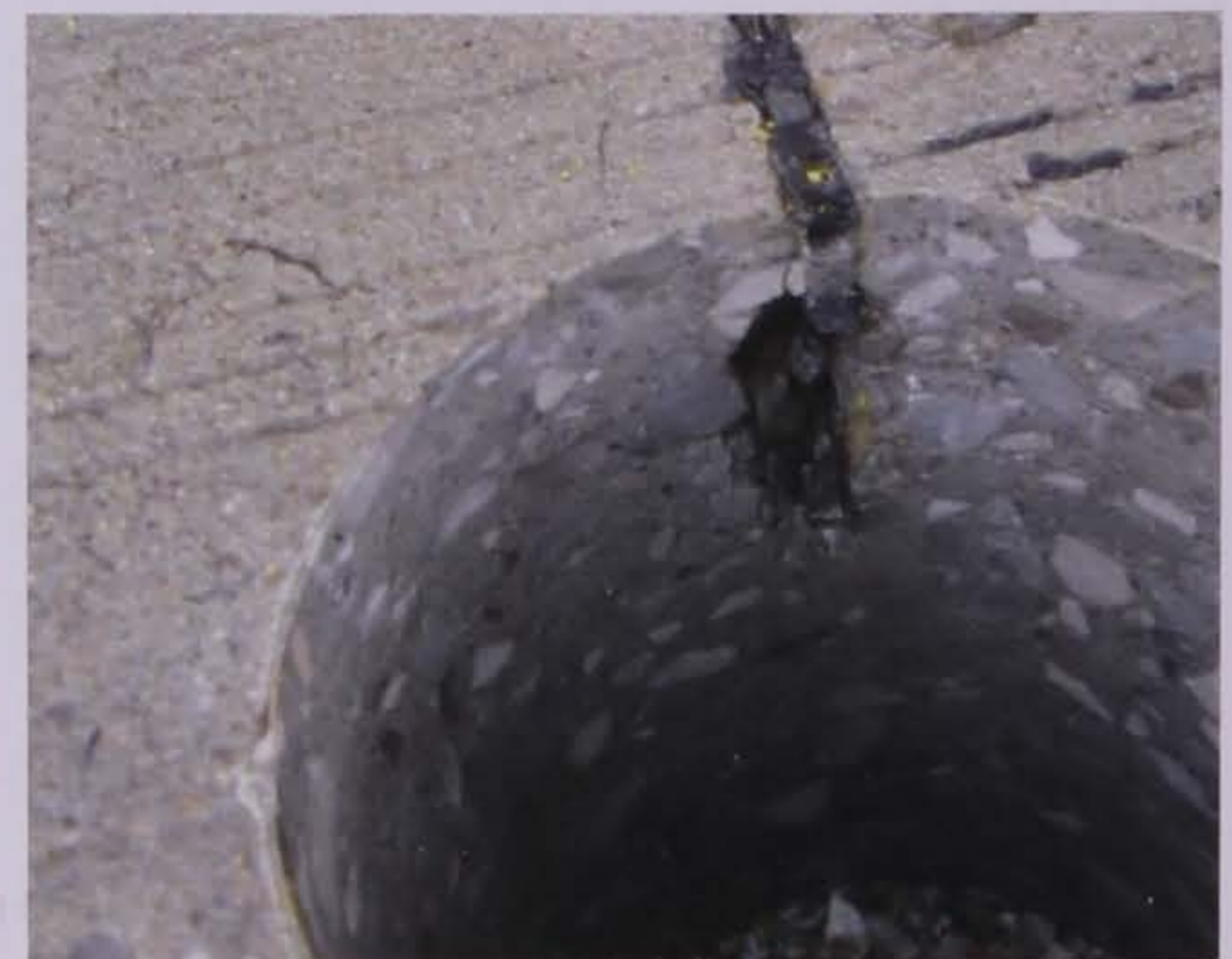
Figure 10.6. Illustration of joint deterioration below the joint sealant (Taylor et al. 2012)
