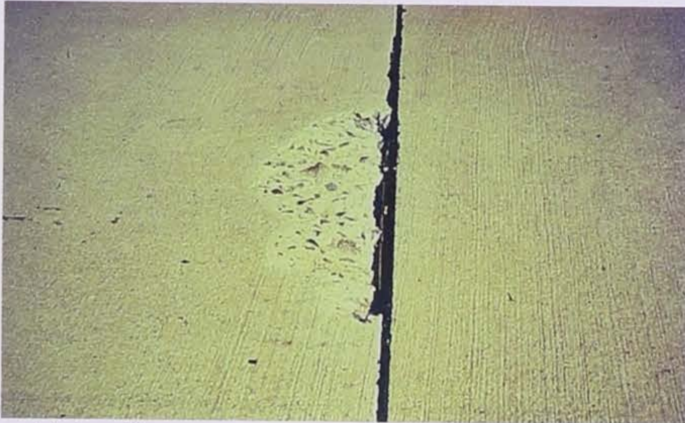
c. Joint spalling
