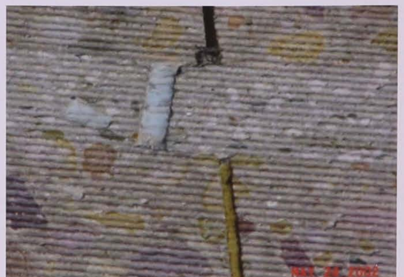
d. Misaligned foam core board
