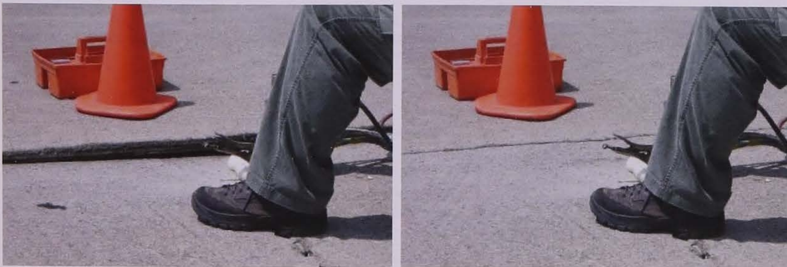
Figure 4.4. Settled slab before (left) and after (right) slab jacking (courtesy of John Roberts, International Grooving and Grinding Association [IGGA])
