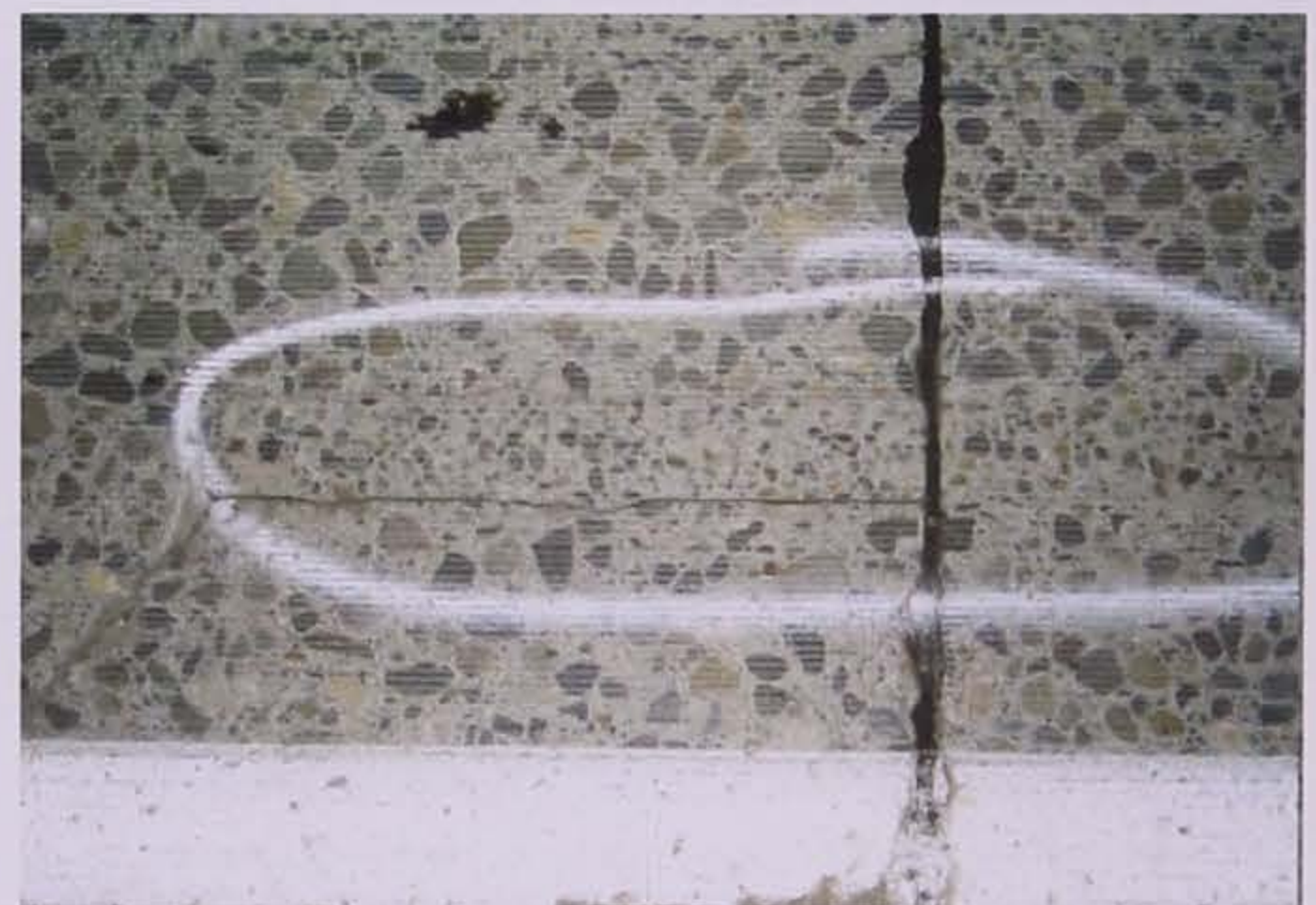
b. Debonding of patching material
