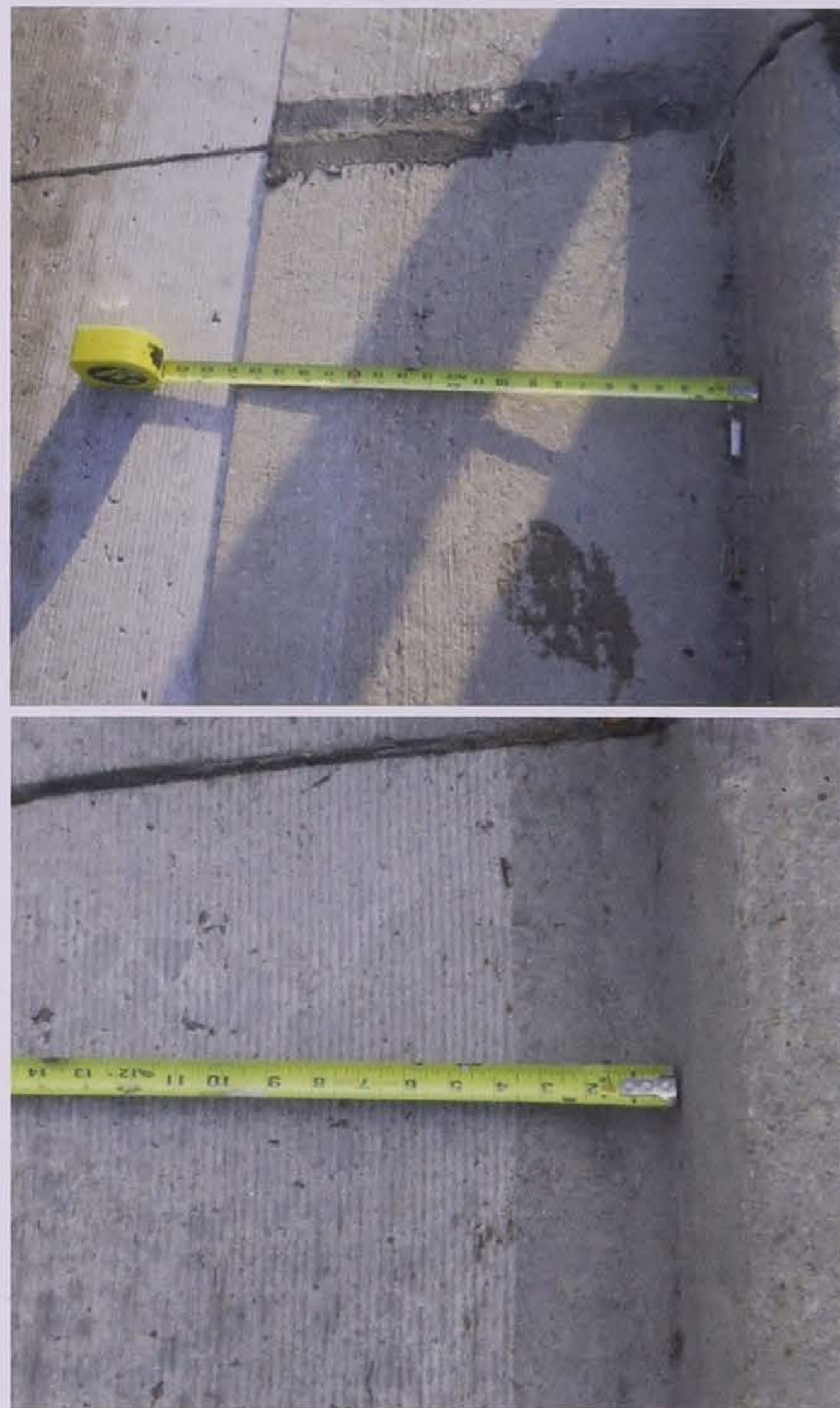
Figure 9.17. Gutter apron before (top) and after (bottom) feathering pass (courtesy of Dan Frentress, IGGA)
