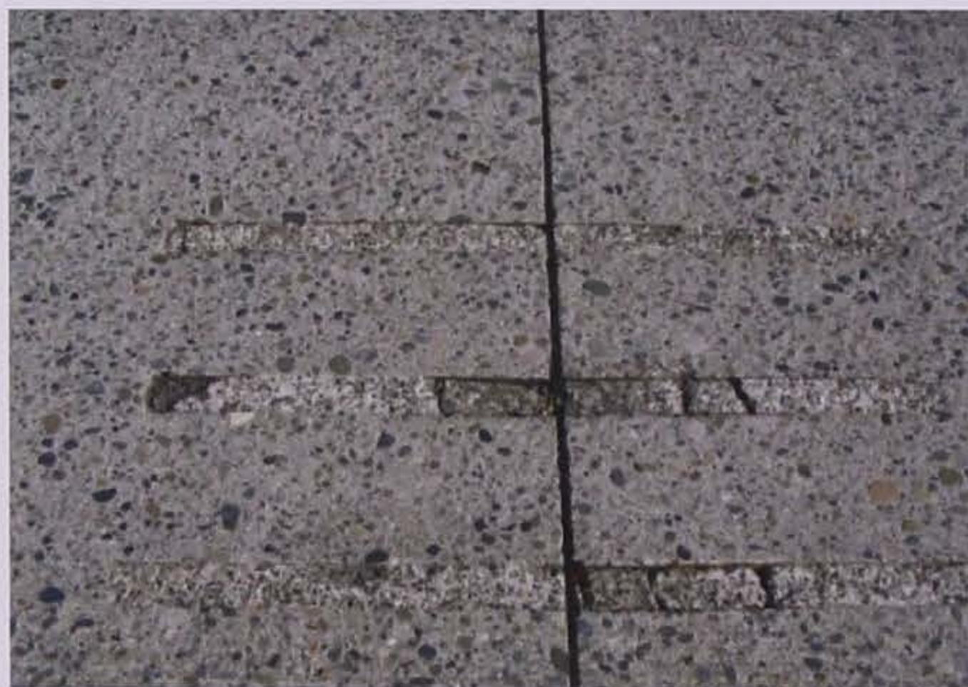
a. Cracking within dowel bar slot
