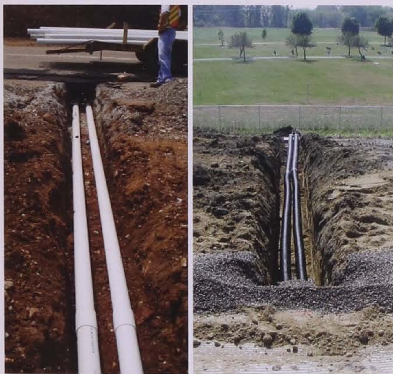
Figure 7.14. Lateral outlet pipes (courtesy of John Donahue [left] and Kevin Merryman [right])
