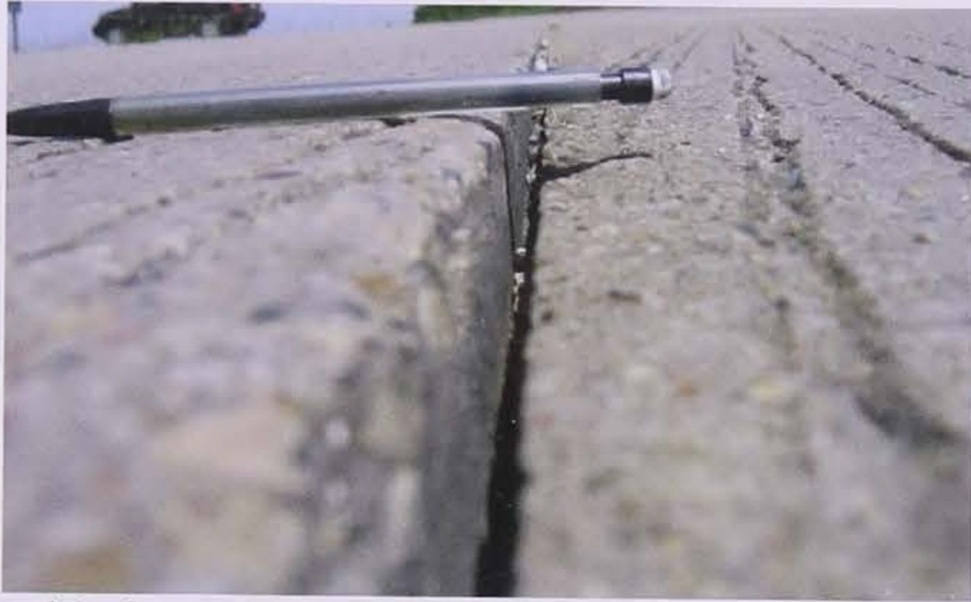
a. Joint faulting
