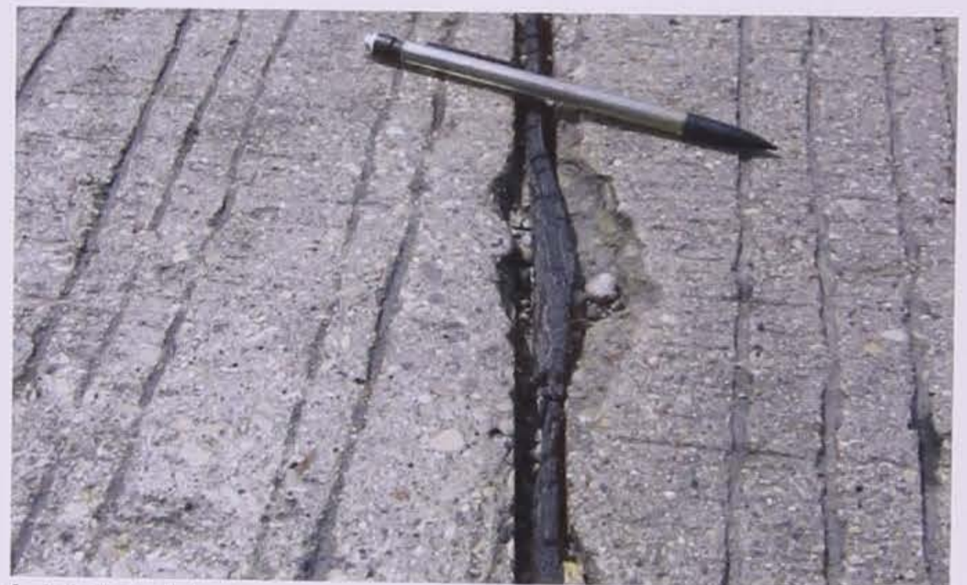
f. Joint seal damage
