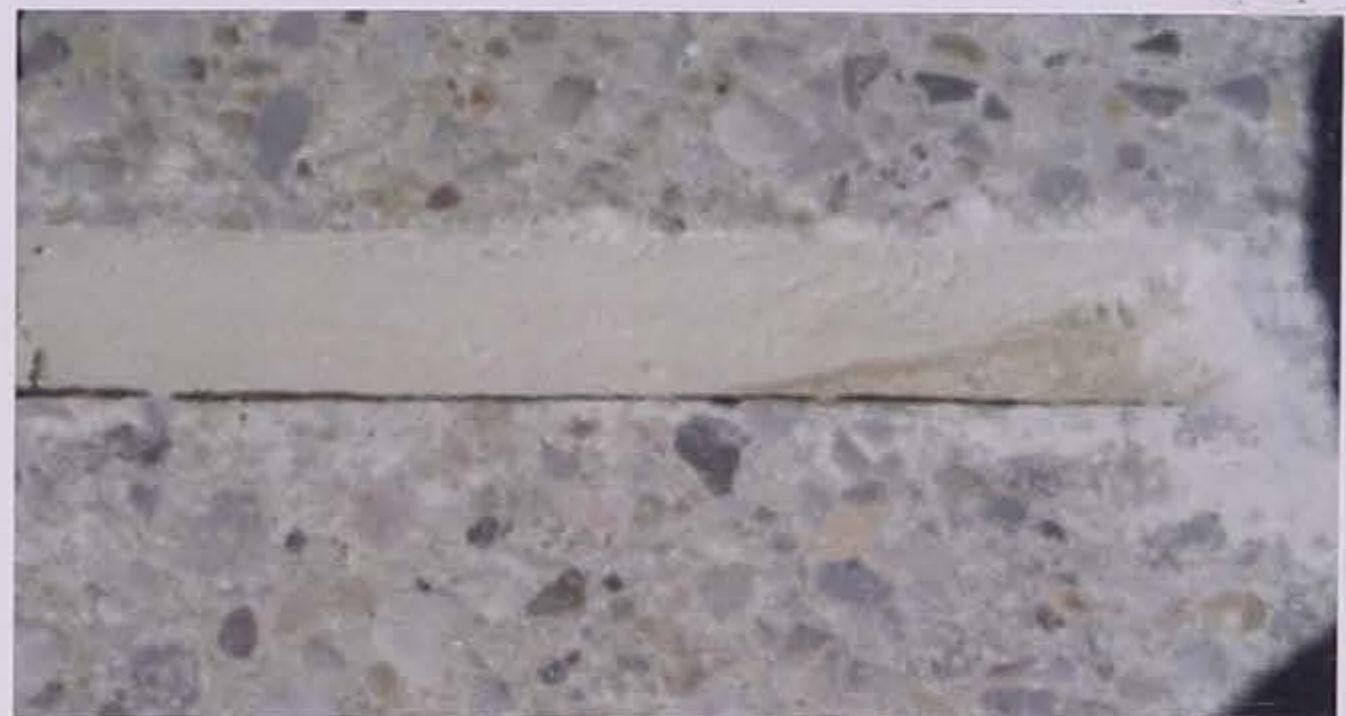
a. Debris and saw blade slurry on side of slot
