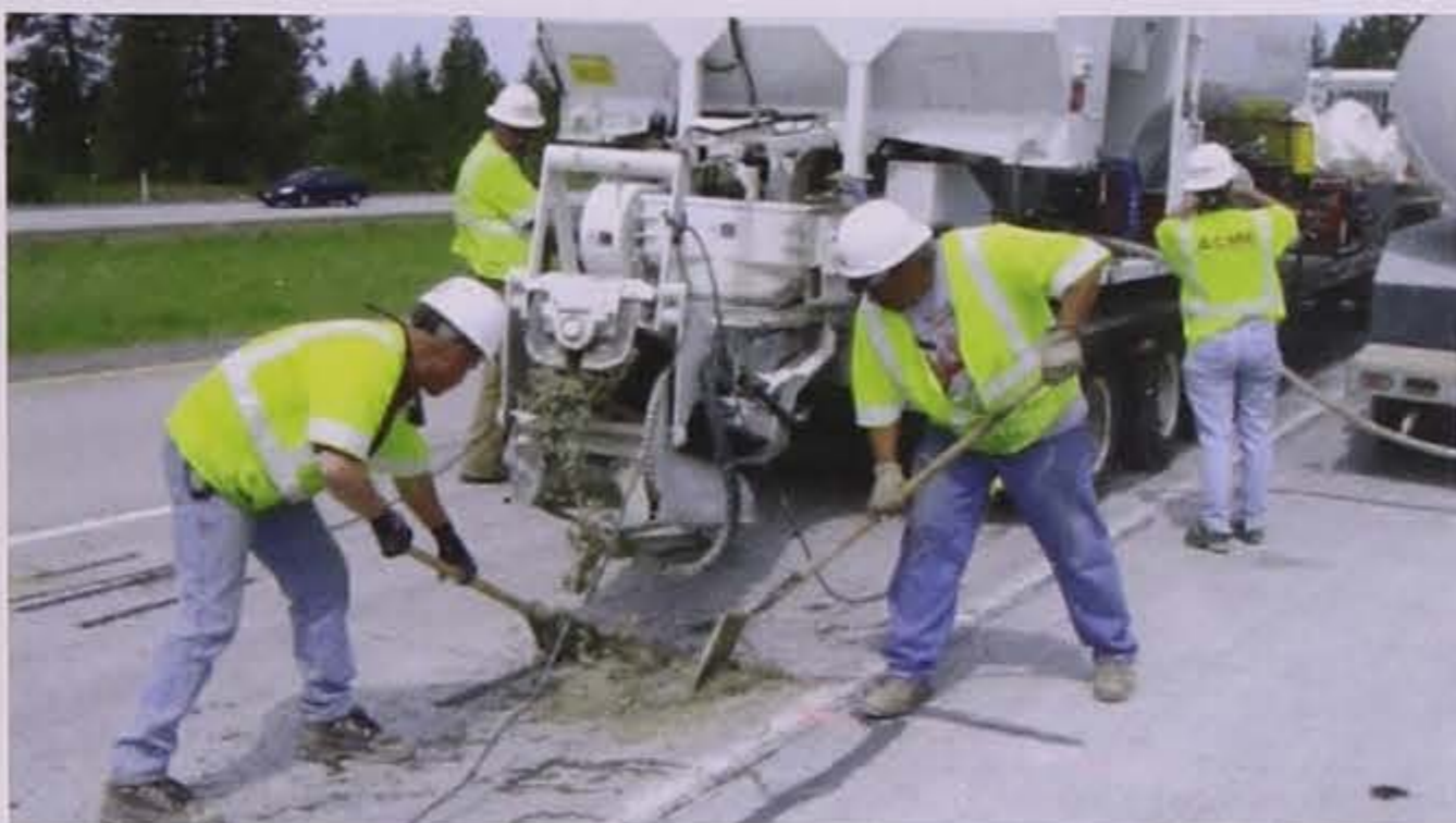
Figure 8.15. Placing patching material into the dowel bar slot (Pierce, Uhlmeyer, and Weston 2009).
