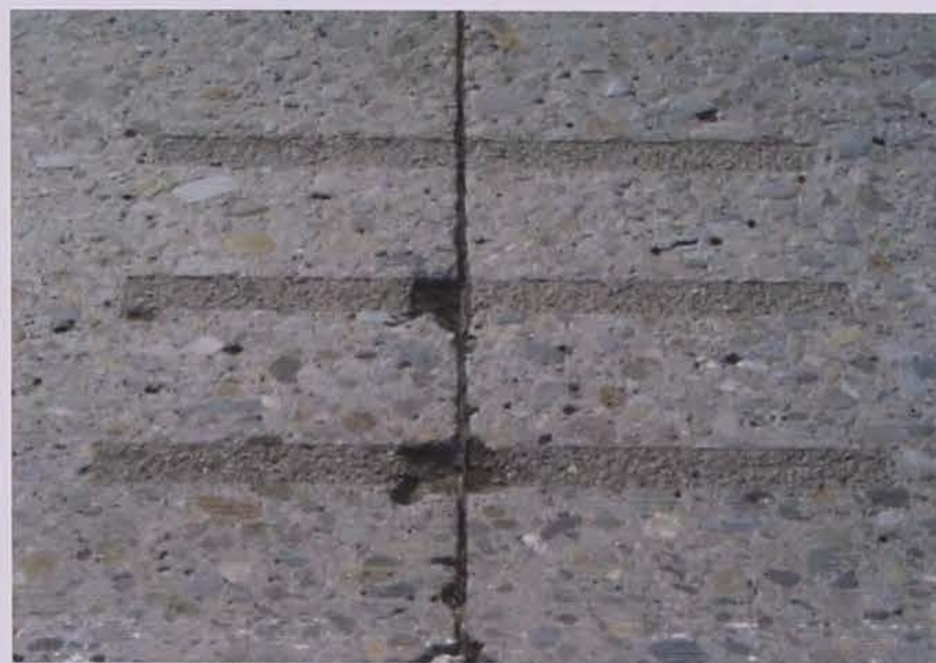
c. Spalling within dowel bar slot
