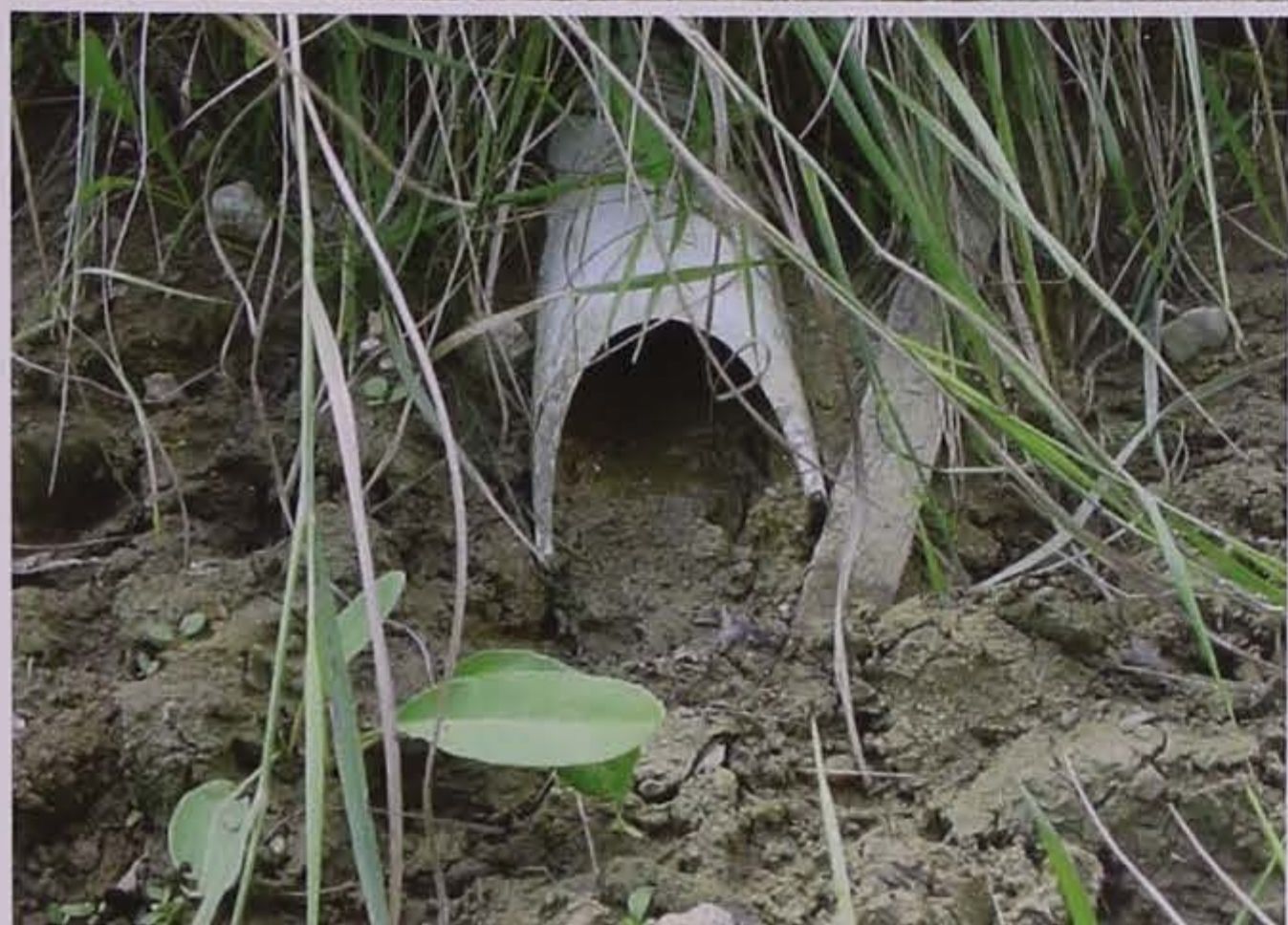
Figure 7.17. Clogged outlet pipes (courtesy of John Donahue)
