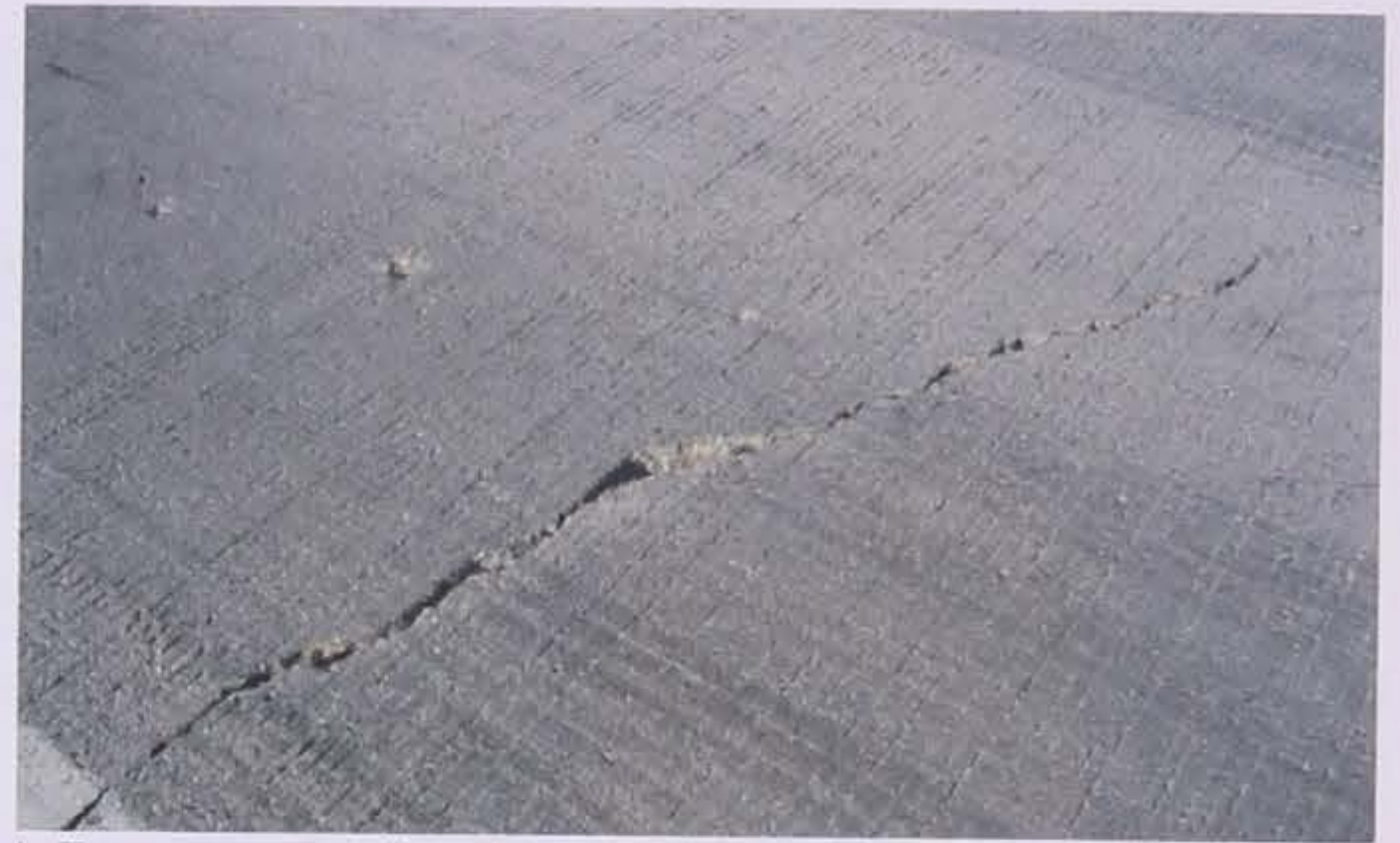
b. Transverse cracking
