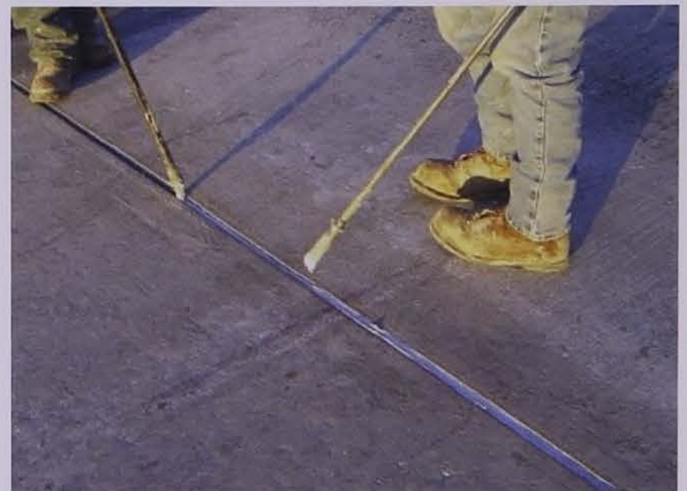
Figure 10.12. Sealant placement at left followed by tooling operation at right (courtesy of John Roberts, IGGA)
