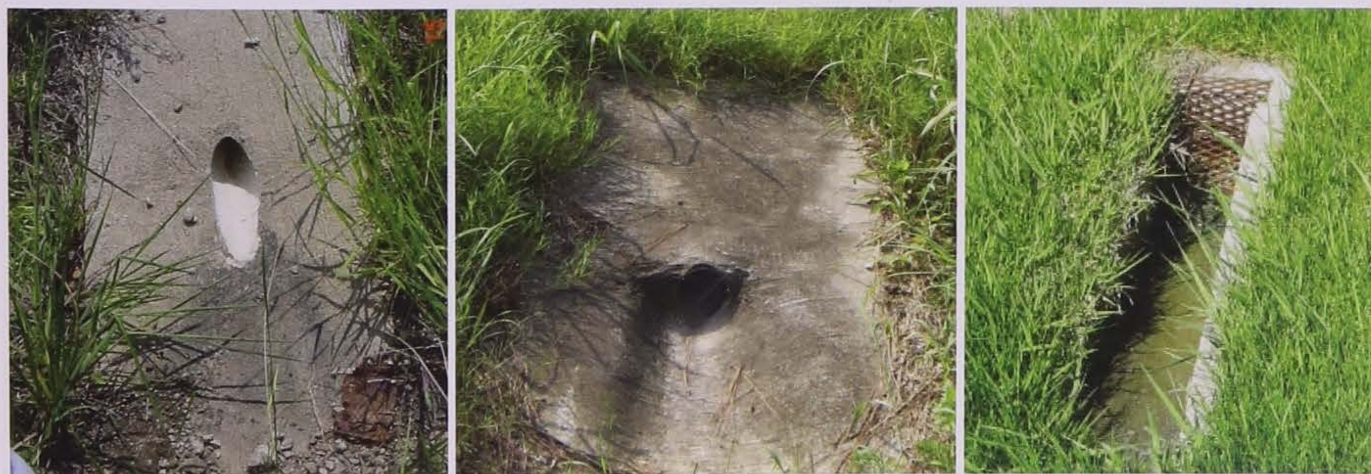
Figure 7.15. Various headwall installations
