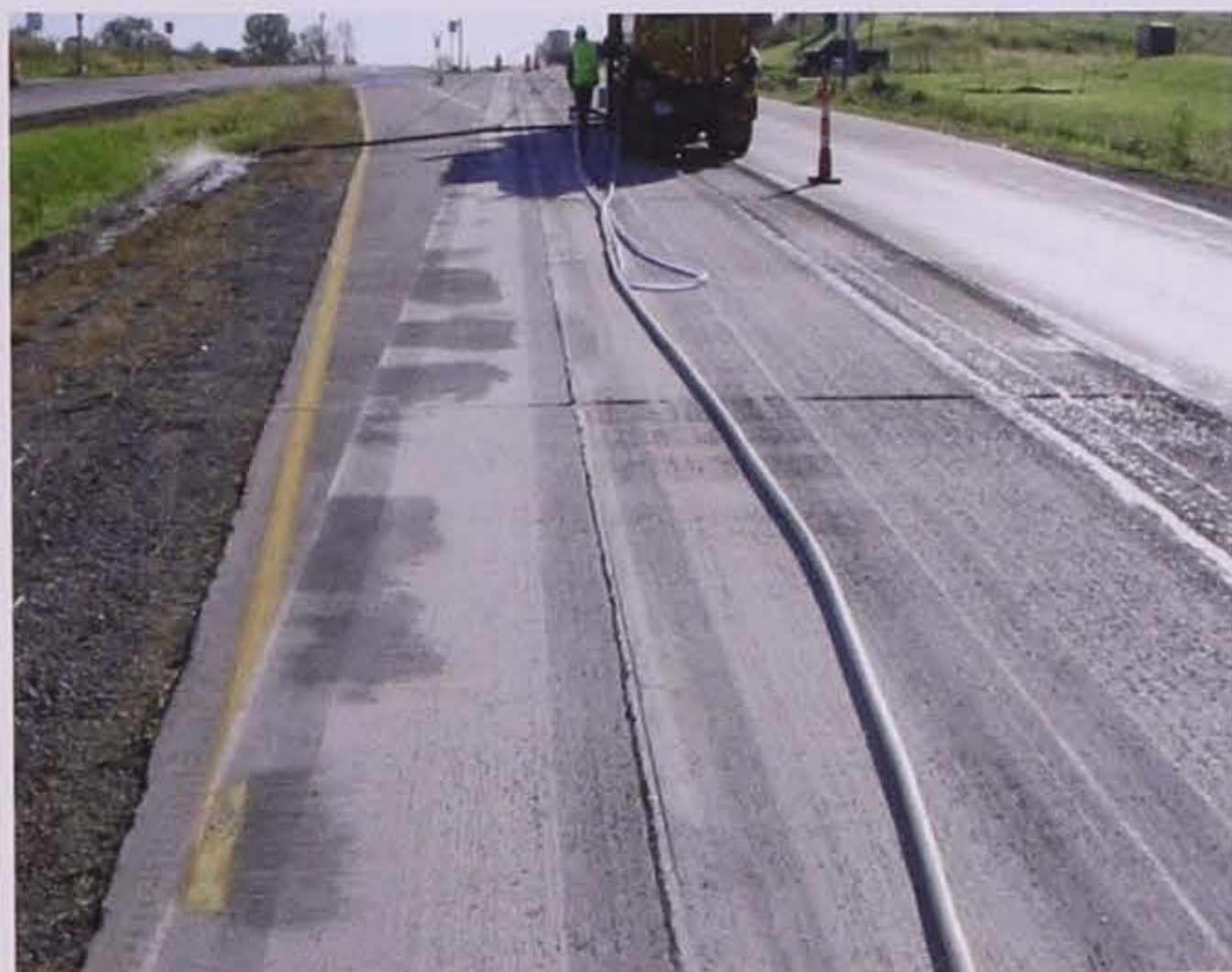
Figure 9.16. Holidays on diamond ground surface of inside turning lane (courtesy of Dan Frentress, IGGA)
