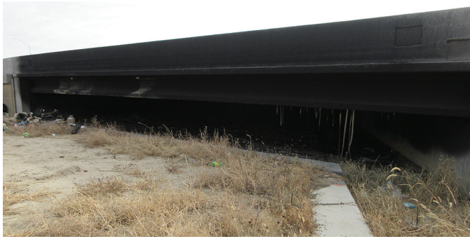
I-29 burned bridge girders over homeless encampment in Sioux City, Iowa
