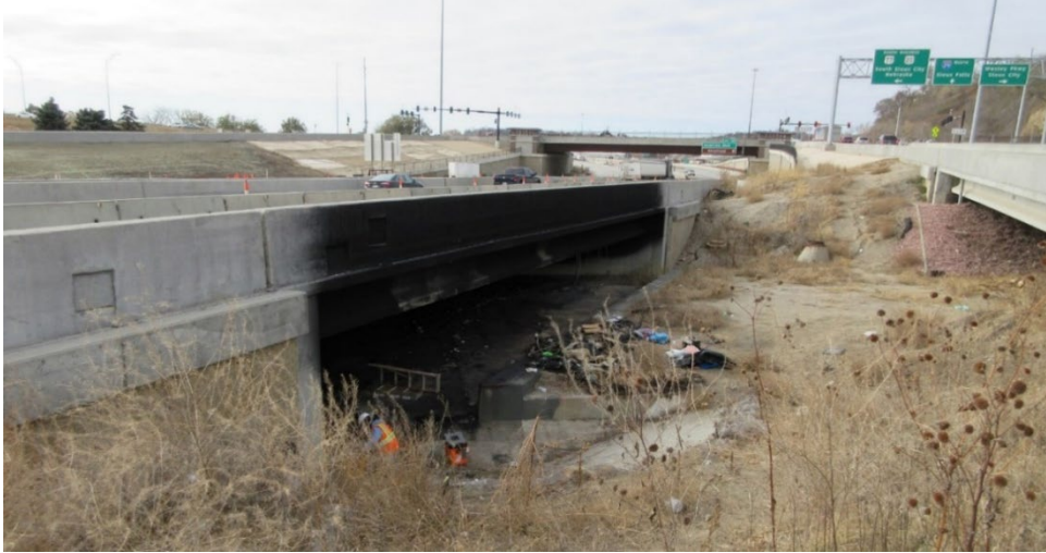
Figure 1. I-29 Bridge fire in Sioux City, Iowa (north side of bridge looking toward west abutment)
