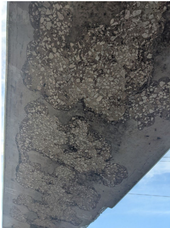
Figure 49. Spalling of concrete on bottom side of Girder G
