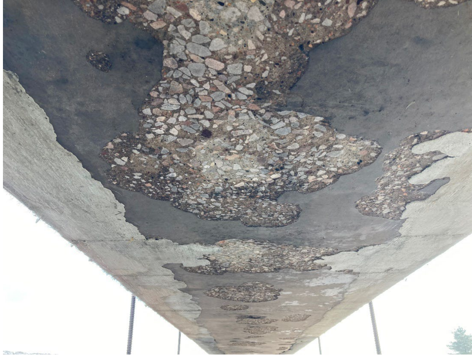
Figure 83. Bottom of girder spalls prior to repair
