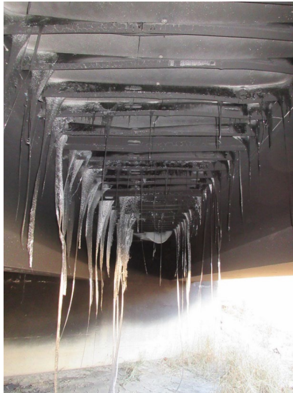
Figure 4. Melted polycarbonate stay-in-place forms
