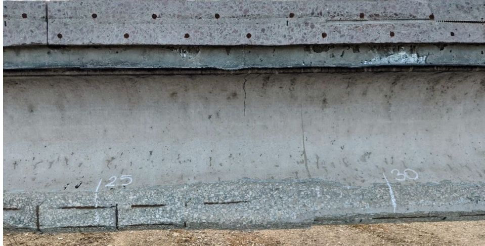
Figure 50. Exposure of steel reinforcement as a result of concrete spalling on Girder G
