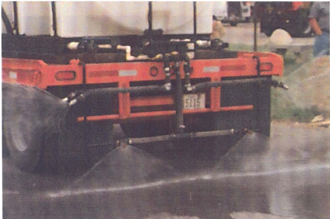
Fan nozzles – Provide complete coverage of roadway
