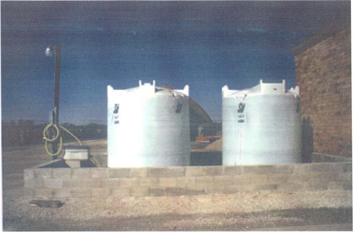
Another example of external storage using block wall construction, external lighting and covered pump
