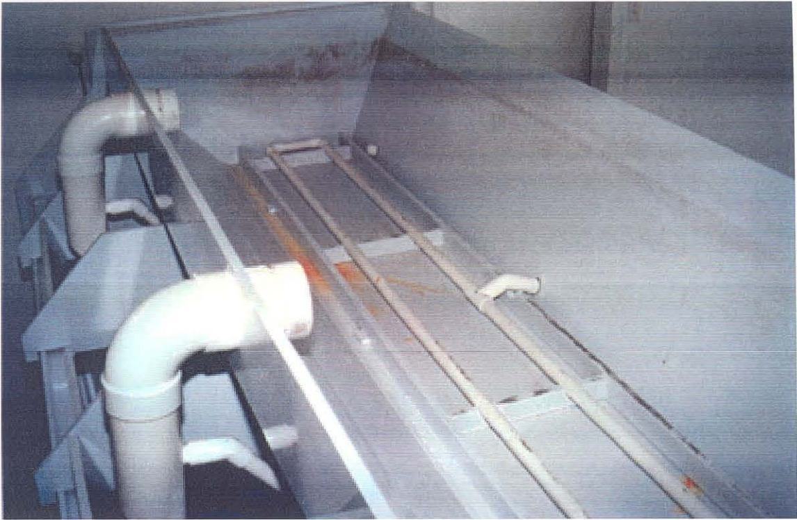
Inside view of Varitech unit – Shows water supply system that percolates water up and through the salt that then overflows as brine into the lower tank.
