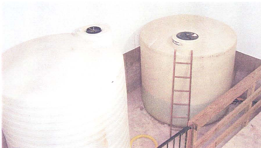
Internal brine storage
