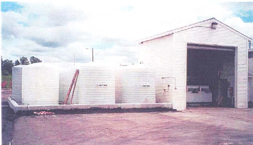
External brine storage with containment
