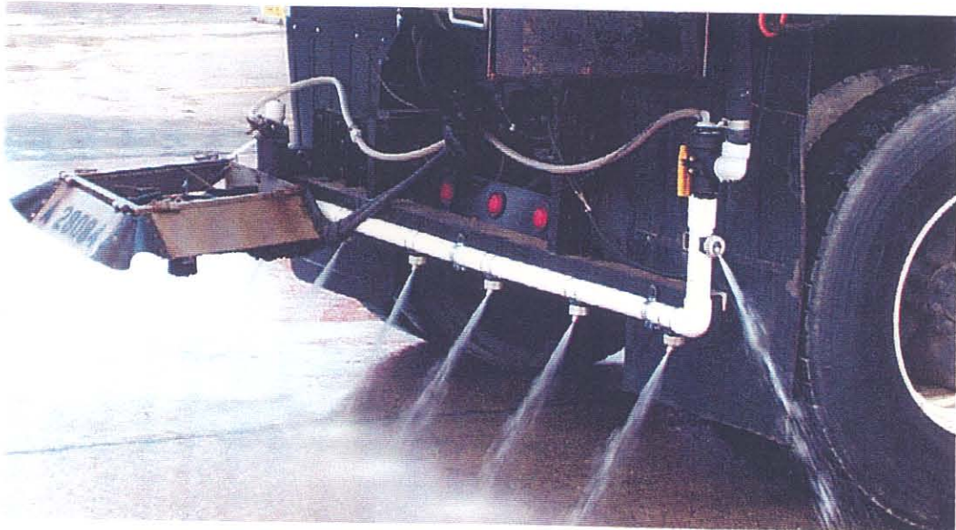
1 ½ inch PVC pipe with clip-on nozzles that can also be converted to prewetting onto the spinner. (Pressure System)
