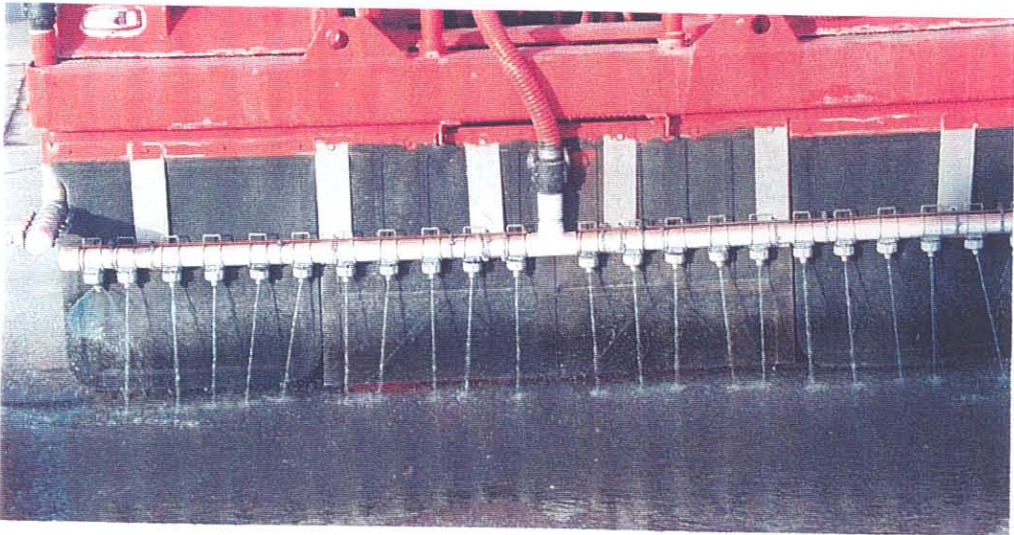
2 inch PVC pipe with drilled holes or clip-on nozzles. (Gravity System)
