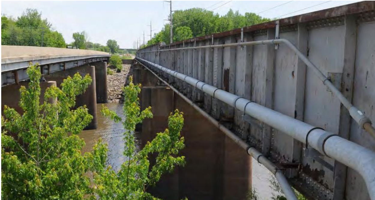
Figure 13 – Fiber Optic and Electric Utility Infrastructure in the CRANDIC Corridor Right-of-Way near Mid-River
