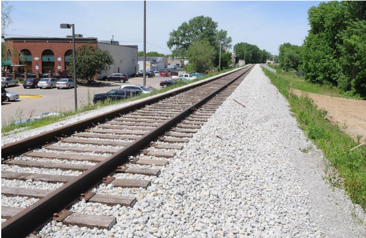
Figure 16. Typical Section of CRANDIC Corridor Right-of-Way at Rocky Shore Drive in Iowa City
