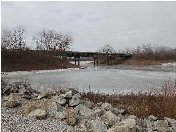
Photo 15. I-380 NORTHBOUND OVER IOWA RIVER/CORALVILLE RESERVOIR (MP 8) (FLOODING, SNOW, BLIZZARD, HIGH TEMPERATURE CHANGE) – LOOKING NORTHWEST FROM BOAT LANDING EAST OF I-380.
