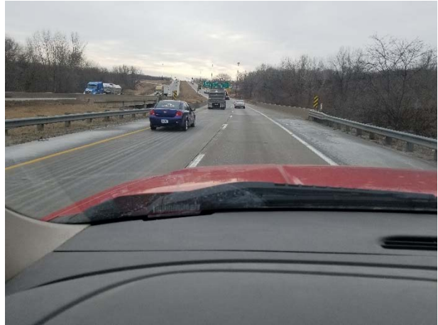
Photo 2. I-380 OVER CLEAR CREEK (MP 0.5) (FLOODING, SNOW, BLIZZARD, HIGH TEMPERATURE CHANGE) – I-380 SOUTHBOUND LANES LOOKING SOUTH
