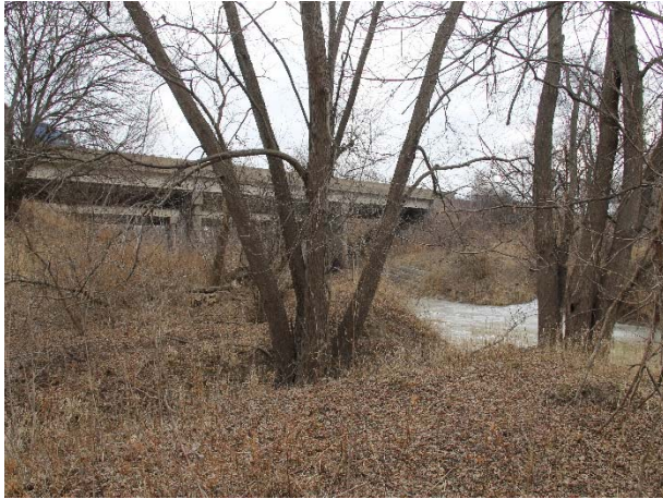
Photo 1. I-380 SB OVER CLEAR CREEK NEAR MILE POST (MP) 0.5 (FLOODING, SNOW, BLIZZARD, HIGH TEMPERATURE CHANGE) – LOOKING SOUTH FROM CLEAR CREEK TRAIL
