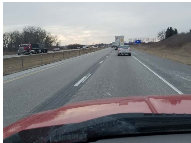
Photo 12. I-380 NEAR MP 6 (FLOODING, SNOW, BLIZZARD, HIGH TEMPERATURE CHANGE) – SOUTHBOUND LANES LOOKING SOUTH
