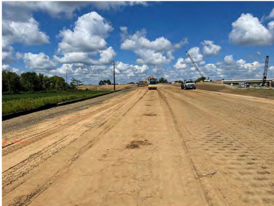
Figure 33. Photo of Subgrade (Sand) on I-380 Ramp C at location of compaction curve mapping.
