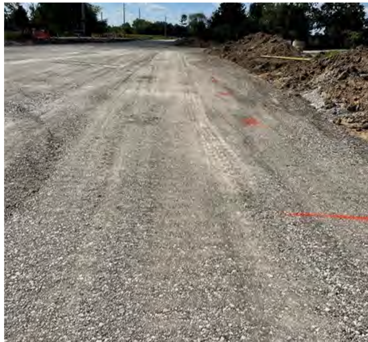
Figure 35. Photo showing Modified Subbase Recycled Composite material on Tower Terrace Road at location of compaction curve mapping.
