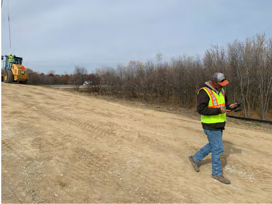
Figure 53. Photo showing Iowa DOT inspector moving around to viewing map data using Comp-Score INSPECTOR.
