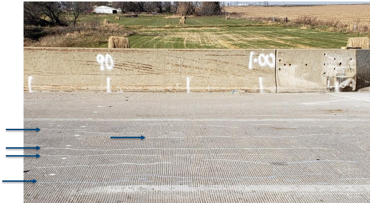
Figure 3.2. Photograph of topside of bridge deck with longitudinal cracking, identified with blue arrows.
