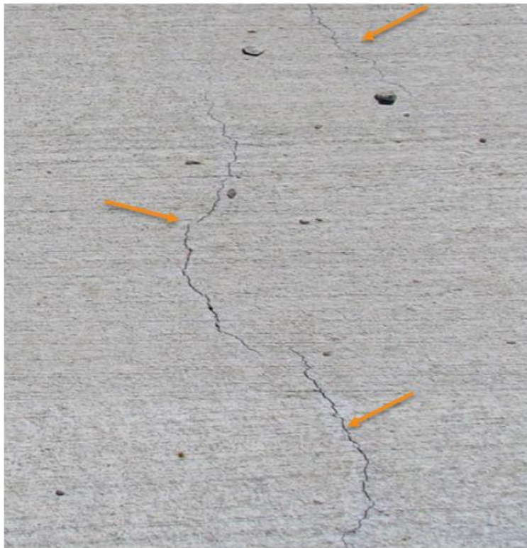
Figure 3.4. Photograph of plastic shrinkage cracks, identified by orange arrows.
