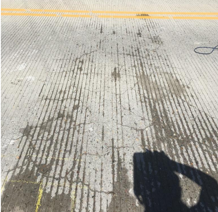
Figure 3.3. Photograph of pattern cracking on a bridge deck.
