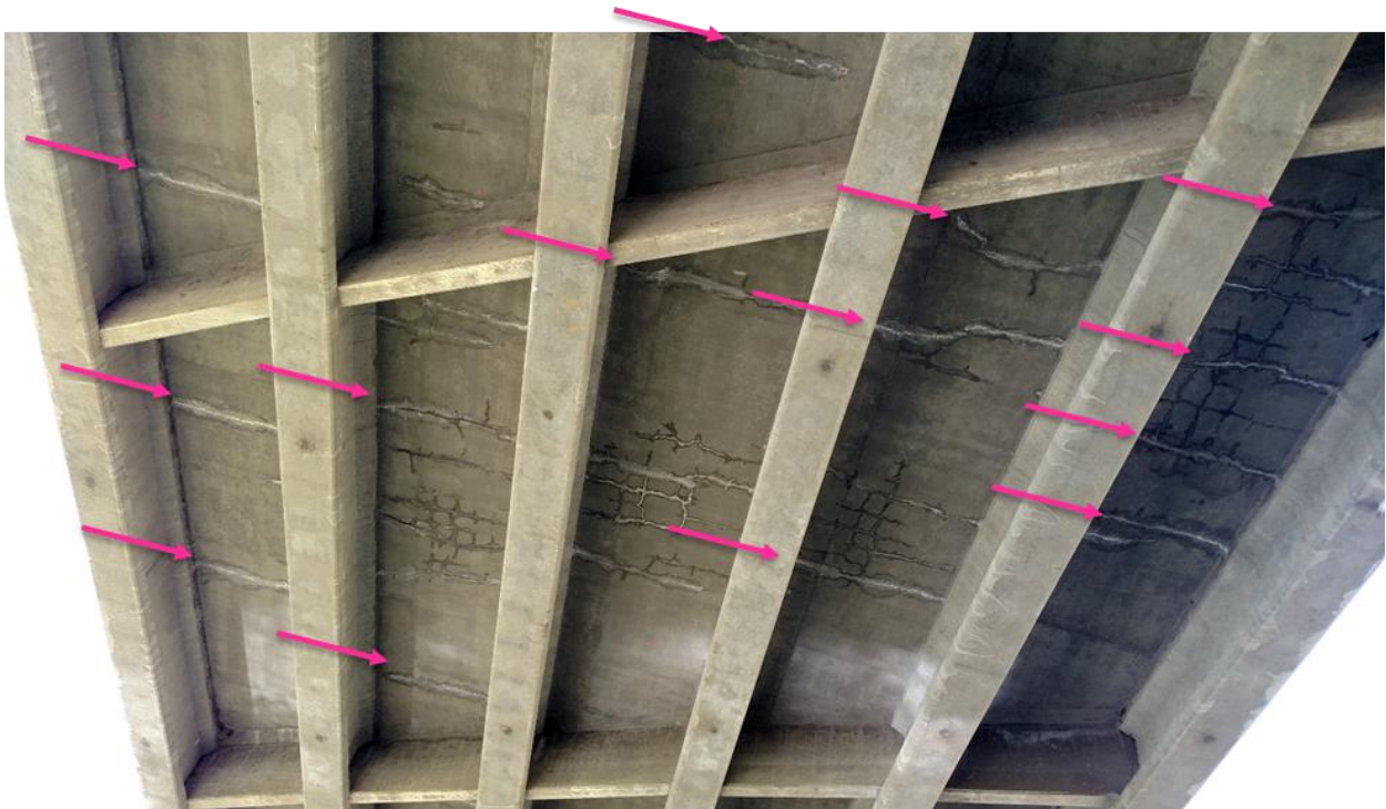
Figure 3.1. Photograph of underside of bridge deck with efflorescing, through-deck cracks. Transverse cracks are identified with pink arrows.
