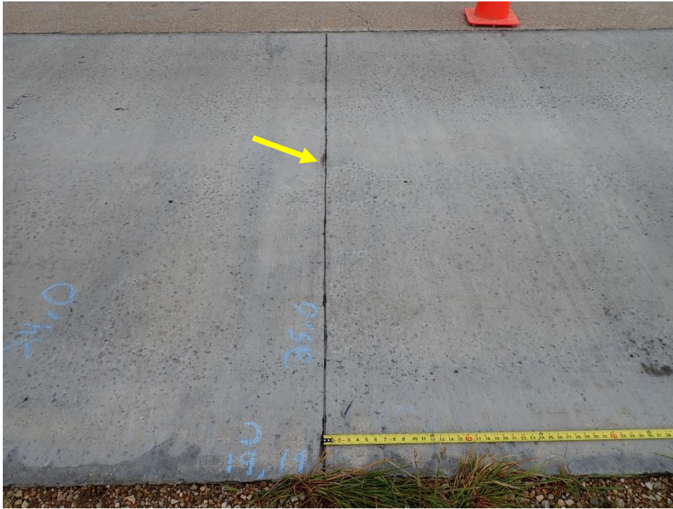
Figure 6.8. Transverse joint exhibiting minor raveling (Yellow arrow). (Patch No. 2)
