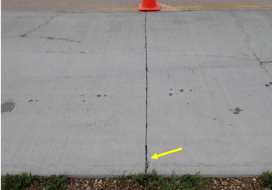
Figure 6.5. Transverse joint exhibiting minor spalling (Yellow arrow). (Patch No. 1).
