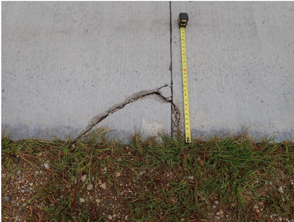
Figure 6.9. Corner break in Patch No. 2, fourth transverse joint from east end.
