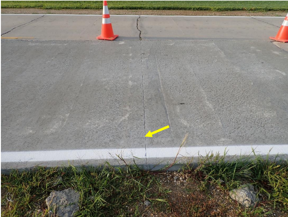
Figure 6.15. Patch No. 4 typical condition. No cracks observed. Transverse joint in good condition with very minor raveling (Yellow arrow).
