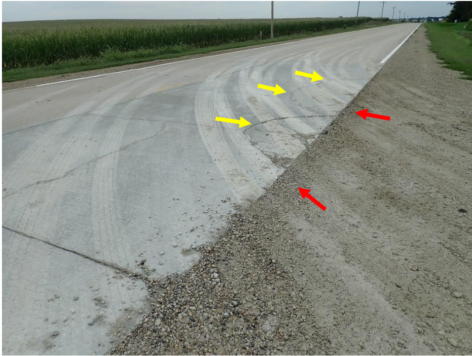
Figure 6.10. Edge and corner breaks (yellow arrows) in wheel paths of vehicles going in/out of M Avenue. Fill materials have loosened and eroded (red arrows).
