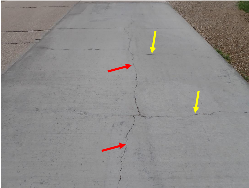
Figure 6.3. Examples of transverse cracks (yellow arrows) and longitudinal cracks (red arrows) in the middle panel in Patch No. 1.
