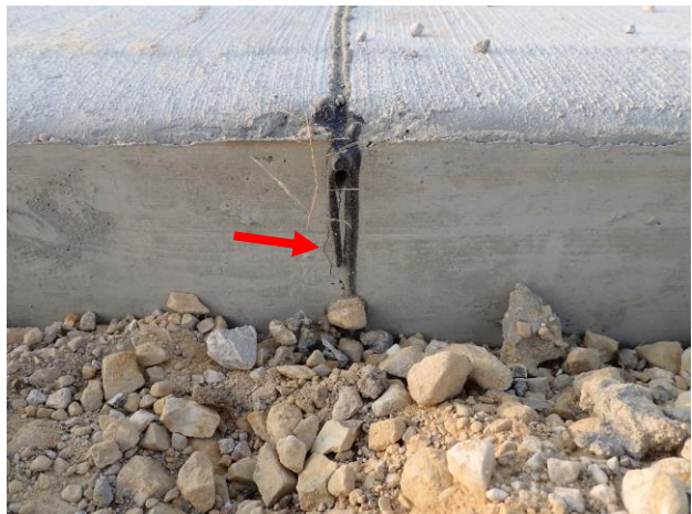
Figure 5.12. Crack formed at transverse joint as expected (Patch 1)
