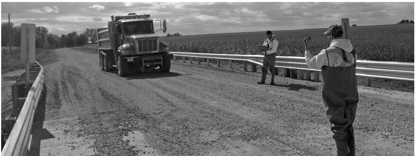
Workers aid in a live load test of the Buchanan County bridge
