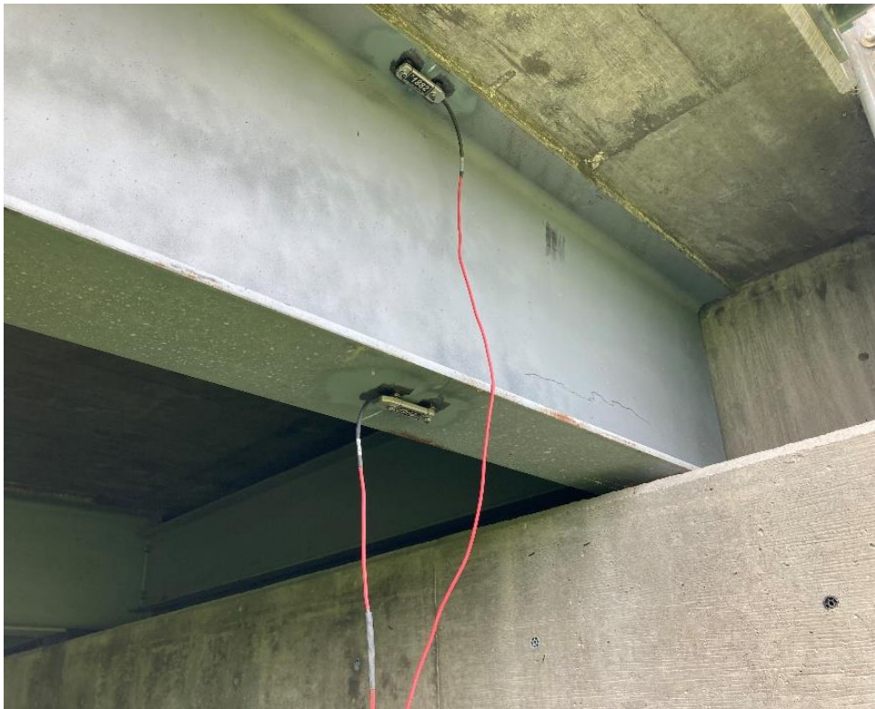
Figure 52. Strain gauges at abutments
