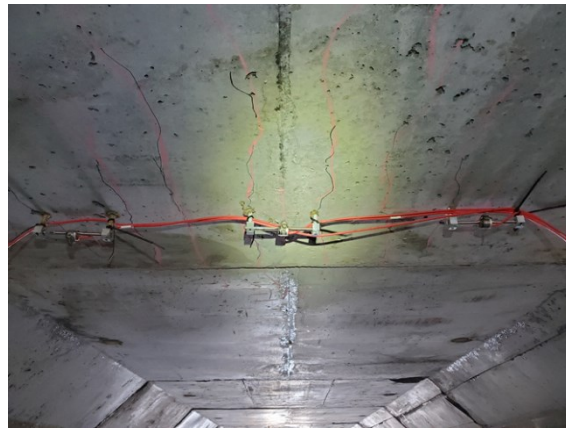
b. Top slab cracking-2
