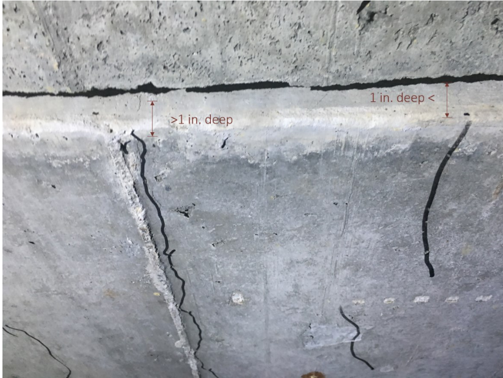
b) Crack depth at the end of instrumented culvert unit
