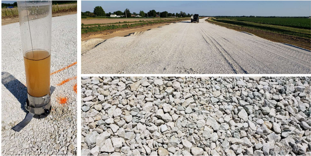
Figure 16. Vu meter testing on crushed limestone granular subbase on Des Moines County US61 project (06/16/2020).
