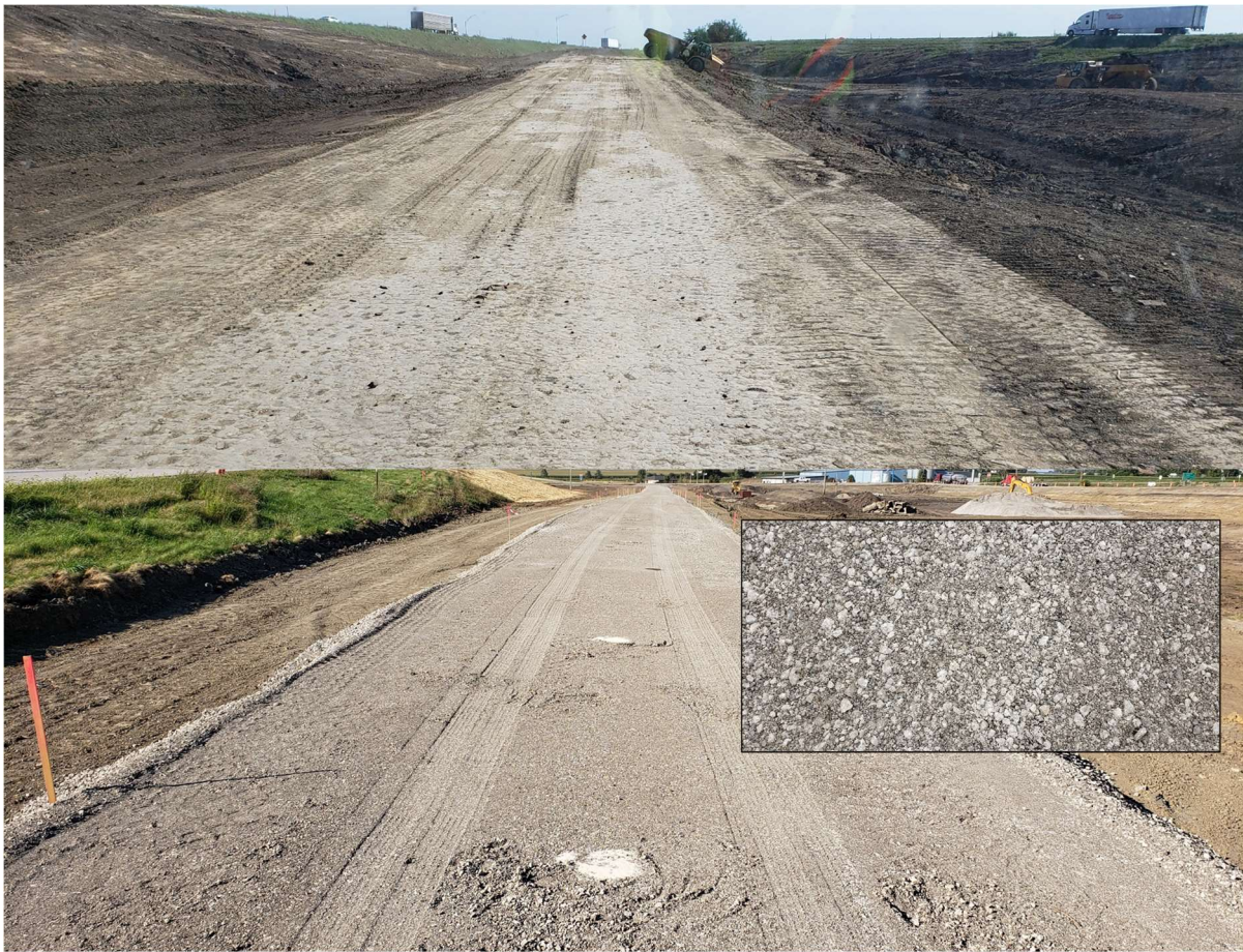
Figure 15. M_{r-comp} map on modified subbase and embankment subgrade Class 10 material on Hamilton County I-35/Hwy 175 project.
