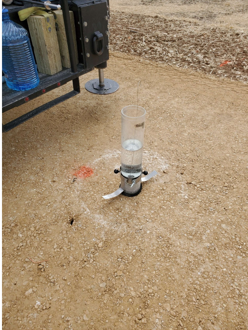
Figure 18. Vu meter testing on crushed limestone modified subbase on Dubuque County US20 project (09/30/2020).
