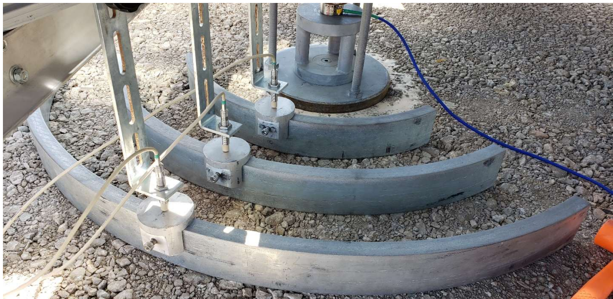
Figure 4. 12 in. diameter loading plate setup for cyclic APLT [picture taken on 08/28/2019 on Blackhawk US20 NHSX-020-6(71)--3H-07 project site over compacted special backfill material]
