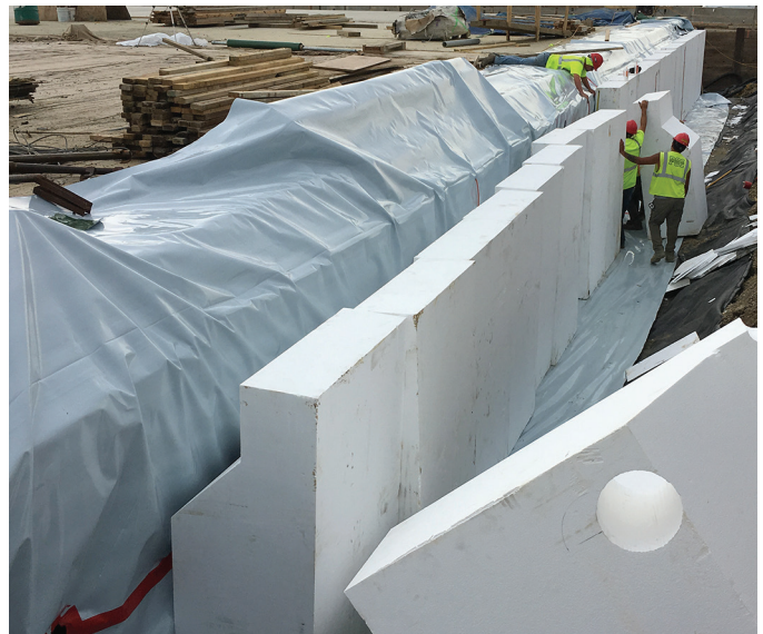
Preparing for placement of expanded polystyrene (EPS) block behind the integral abutments to create thermal isolation from the adjacent backfill soils
