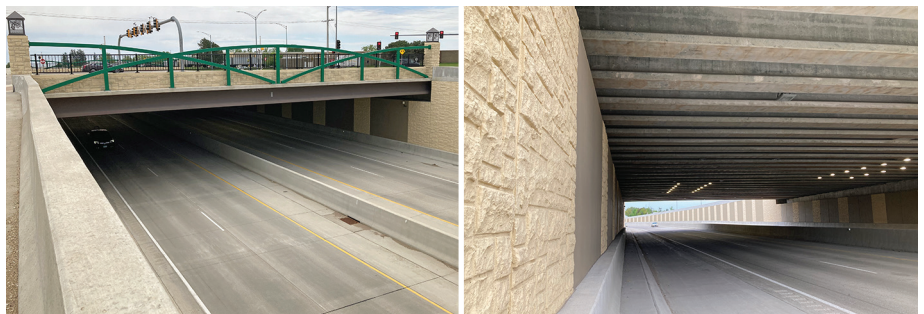
Wide integral abutment Viking Road Bridge over IA 58 constructed with a thermal isolation barrier and without longitudinal expansion joints
