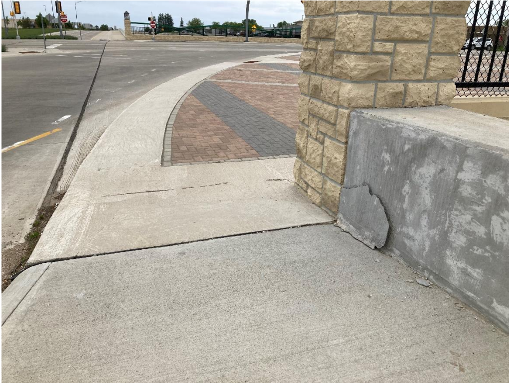
Figure 42. Spalling of rail at northeast corner
