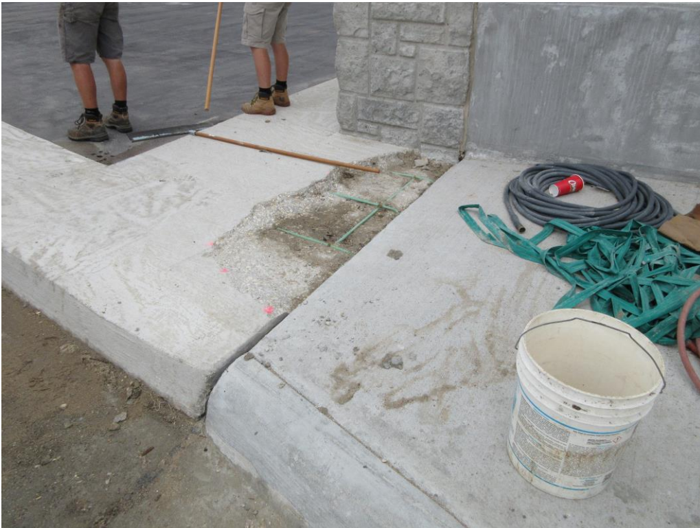
Figure 44. Raised island spalling and repair
