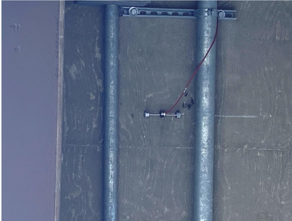
Figure 19. Vibrating wire strain gauge on the deck bottom
