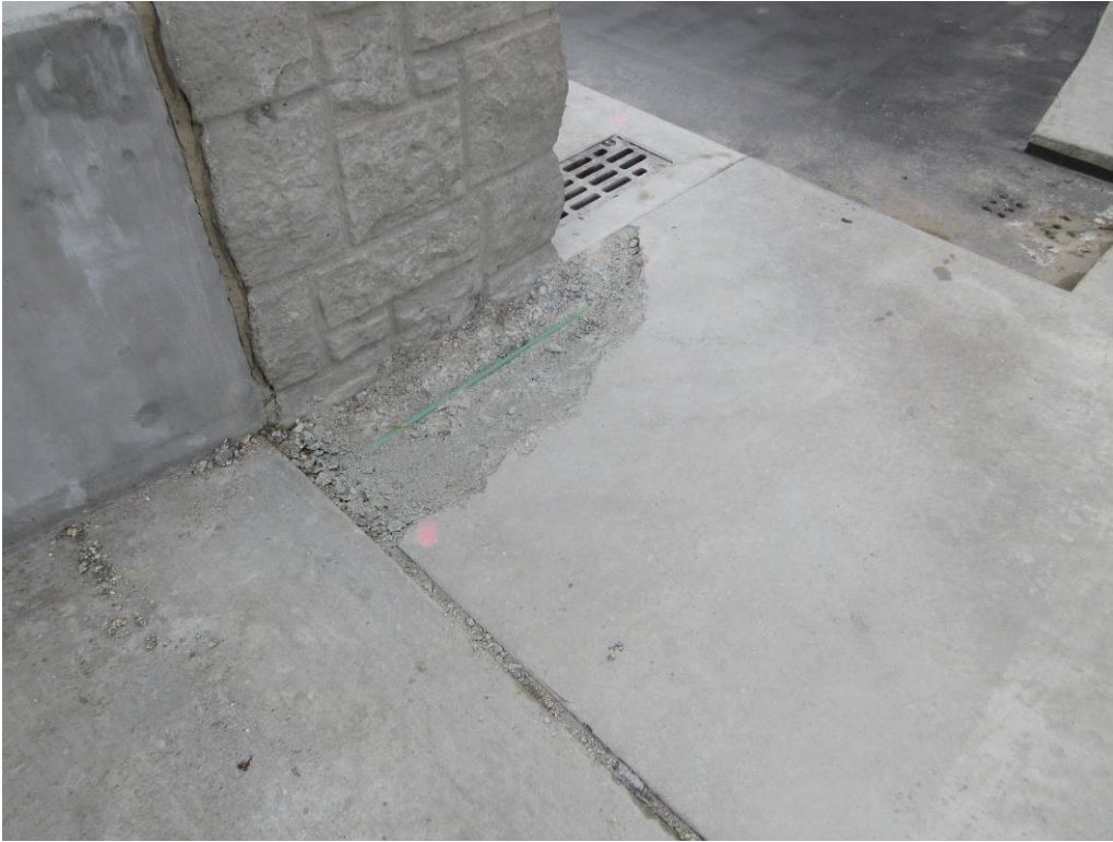
Figure 43. Raised island spalling
