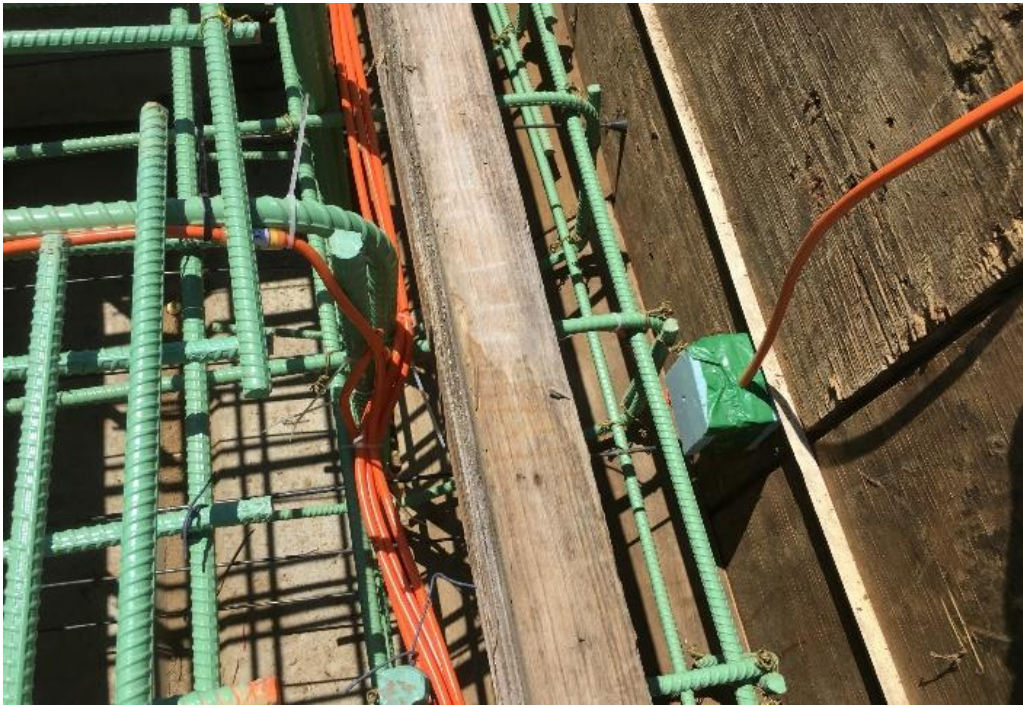
Figure 15. Thermistor placement in deck and at back face of abutment
