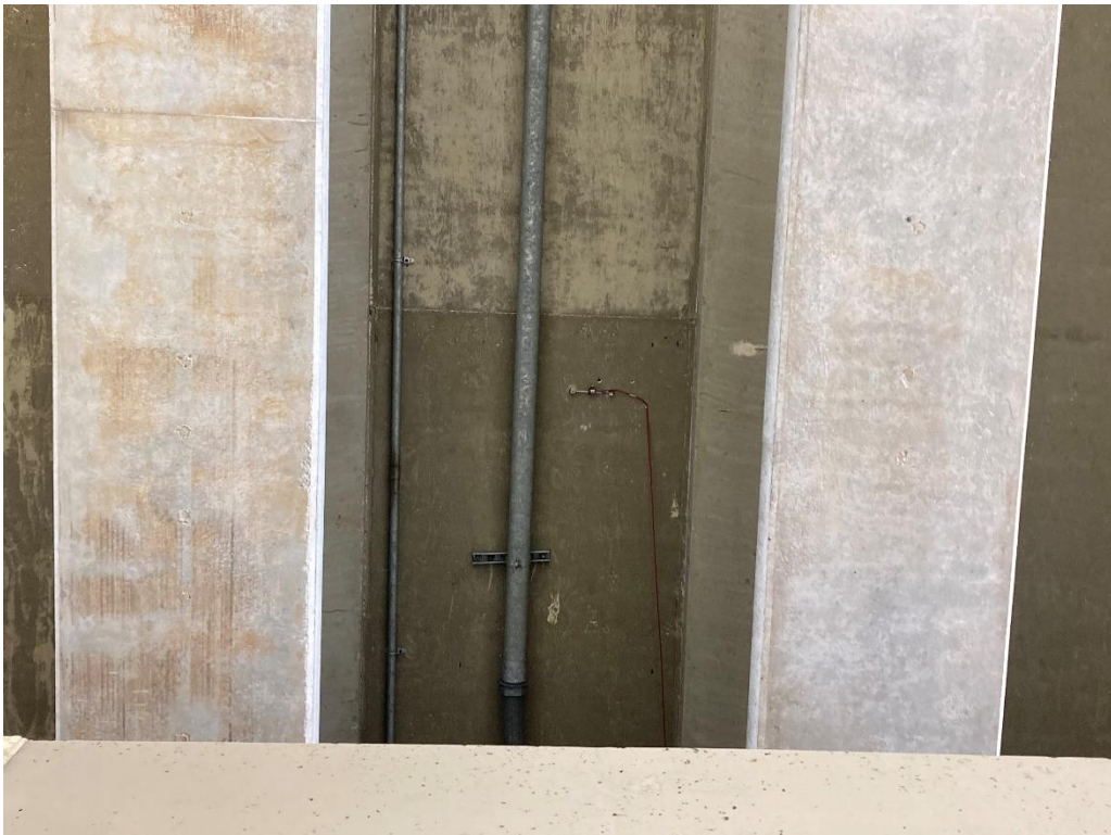
Figure 39. Deck inspection May 2022 Bay JK
