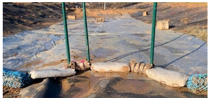
Flocculant blocks in inflow channel
