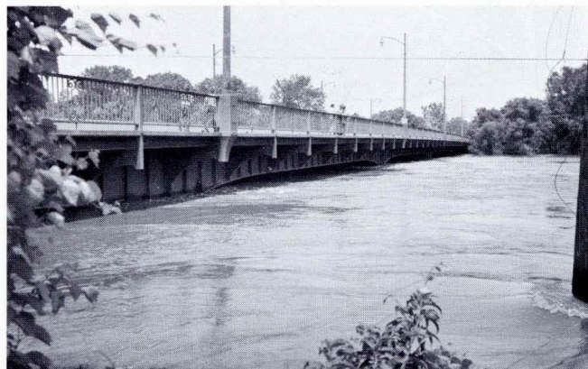
Looking north at the Second Avenue bridge — June 24, 1954 flood.
