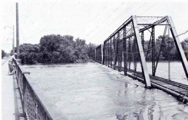
Looking northeast at the D.M. & C.I. R.R. bridge downstream of Second Avenue — June 24, 1954 flood.
