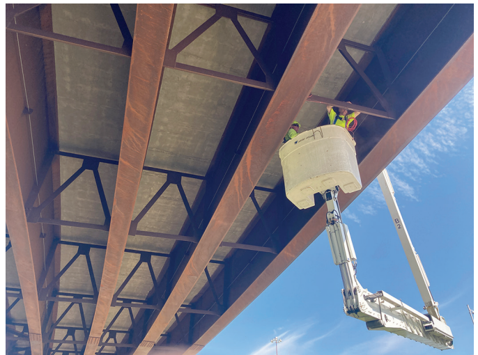
Installation of a strain gauge on the Story County bridge for live load testing
