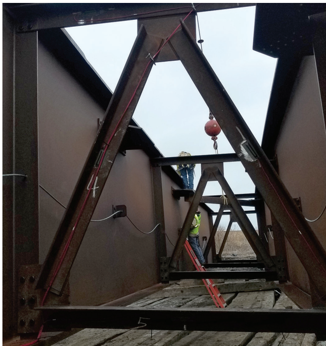
Strain gauge installation on a cross-frame of the Story County bridge for long-term monitoring
