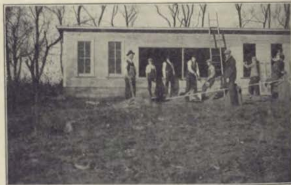
Class in Vocational Agriculture Constructing a Poultry House. Delphos Consolidated School, Ringgold County.
