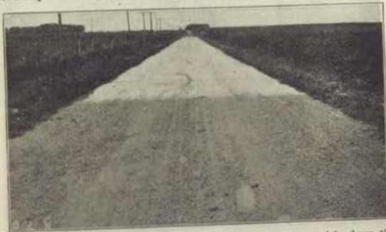
View of Mason City-Clear Lake concrete road. In the background is shown the original concrete surface and longitudinal cracks which have formed under traffic. These cracks are maintained by filling with tar or asphalt, which protect them from wear under traffic. The bituminous top coat has been applied to this road for experimental observation.
