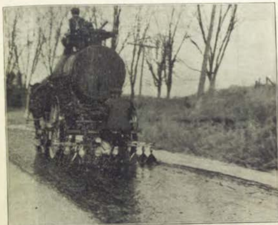
Applying oil with a specially designed distributor. The method of applying the oil is equally as important as the quality of the oil itself. Improper and careless methods of application and a lack of a thorough preparation of the road bed vitiate results obtained, even with the very best quality of oil.
