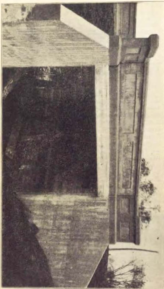
One hundred and thirty-eight bridges of this type were constructed in the state during 1915 at an average cost of $1,200 each. This bridge is located in Cedar county.
