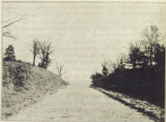
Improvement of Hawkeye Highway in Dubuque county. Showing a 12' rock cut one mile east of Dyersville. The sub-grade has been prepared and rolled ready for the gravel surfacing. It cost 95c per cubic yard to make this cut.
