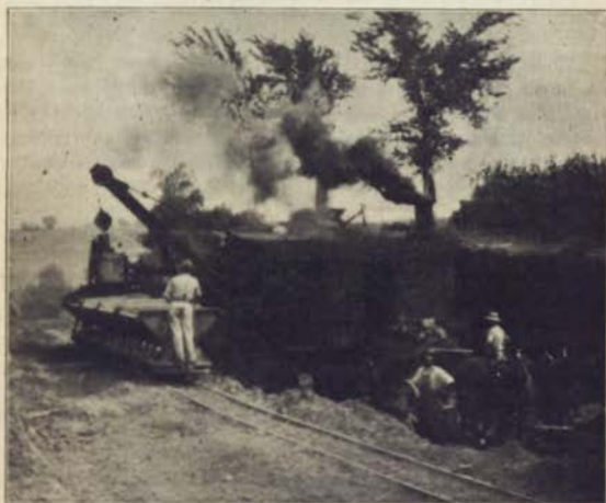
State Road Work. Steam shovel making a 19-foot cut on the North Road at the Iowa State College at Ames. The steam shovel with an engineer, fireman, and water boy, was hired from a contractor. The rest of the work was done by convicts from Anamosa. The dirt was loaded into steel dump cars in trains of five cars each, which were allowed to run down hill under the guidance of a convict brakeman. The empty cars were then drawn back by horses.
