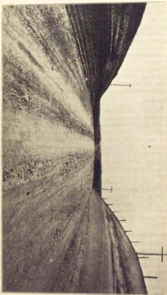
Cut on Des Moines-Keokuk road in Crawford county; 21,000 cubic yards of earth moved on this mile at a unit cost of 18c per cubic yard. Here is a permanent improvement.
