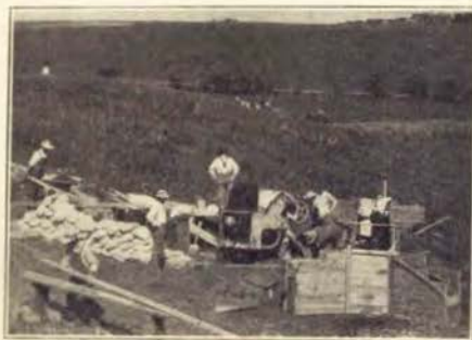
Crew of convicts building a culvert at State Hospital for Insane at Cherokee. This culvert is on the new routing of the Hawkeye Highway through the State Farm of the institution.
