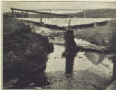
This is typical of the old type wooden culvert built in Iowa under the old system of road and bridge building. This is a culvert on the state farm at Woodward which has since been replaced by a concrete box culvert.
