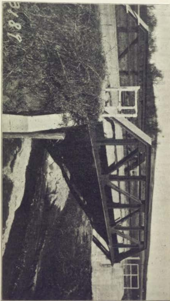
This is a typical (X series) low riveted steel truss span with concrete floor and abutments. Located in Crawford county.
