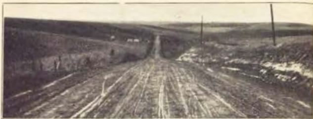
Typical mile of permanent grade constructed during the 1915 season in Crawford county. This mile is on the Soldier-Dunlap road.
