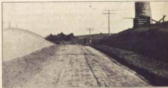
Improvement of Hawkeye Highway in Dubuque county. Earth cut east of Farley. Note the care with which the side slopes have been shaped. The sub-grade has been rolled ready to receive the gravel surfacing. It cost 20c per cubic yard of earth to make this cut.
