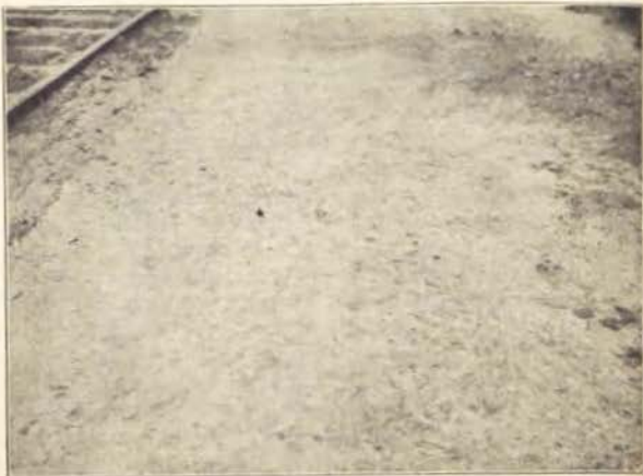
Faulty concrete pavement surface—improper consolidation of the concrete, the use of soft and friable aggregate, in many cases covered with a coat of finely divided clay or dirt, together with a mortar which was too lean to withstand abrasion, has resulted in a surface of this character. The mortar carpet has rapidly scaled away, and the stones are picked out piece by piece, due to faulty bonding of the material in the concrete.
