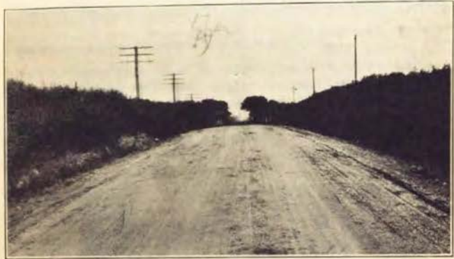
This view shows a finished section of the experimental mile of two course gravel road built on the Hawkeye Highway just east of Ft. Dodge during the season of 1915.
