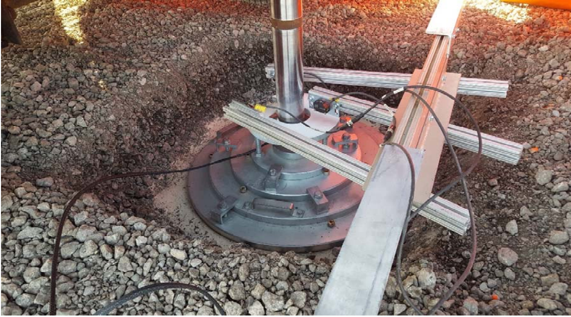
Figure 10. 30 in. diameter loading plate setup for static APLT on Project 2 - US 20 (picture taken on 10/19/2017).
