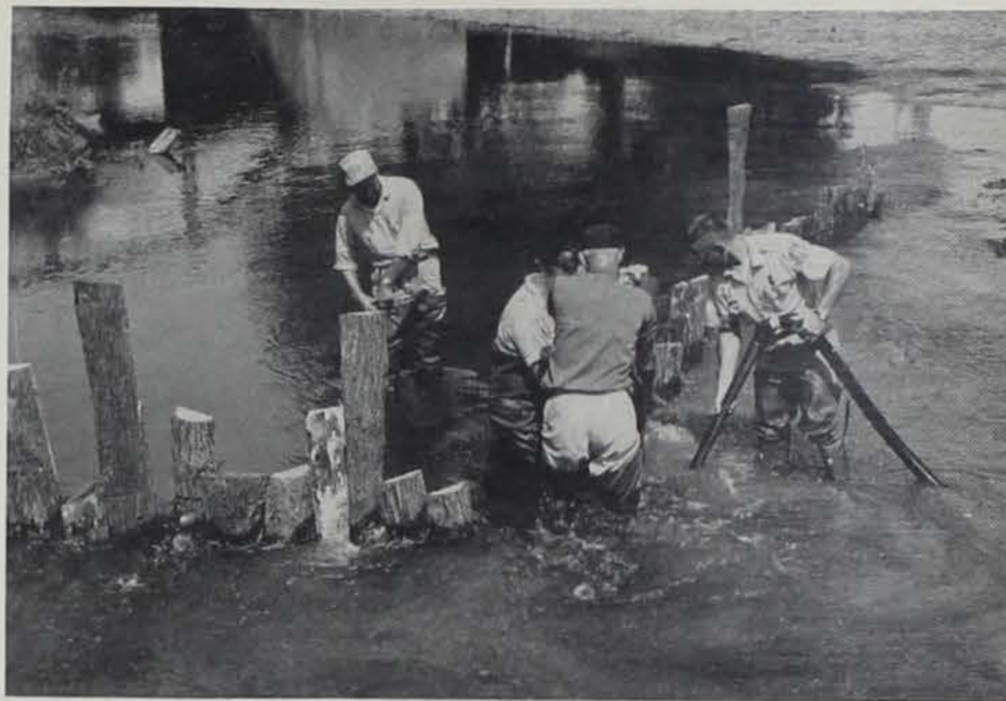
At an installation demonstration in August, Chickasaw County Conservation Board members demonstrated the ease with which their stream improvement device can be installed. The water was six inches deep before installation of the structure.
