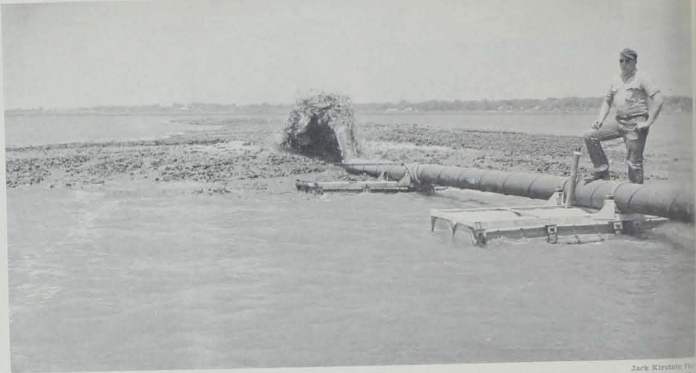
Out in Storm Lake the dredge pumps away, building the first of a series of islands. The mudballs used to raise the ring dike are easily seen here.
