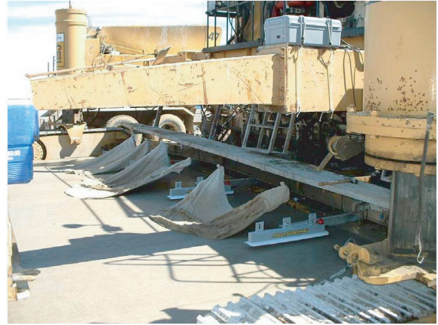
Measuring pavement profile during construction using the Ames Engineering Real Time Profiler (RTP)
