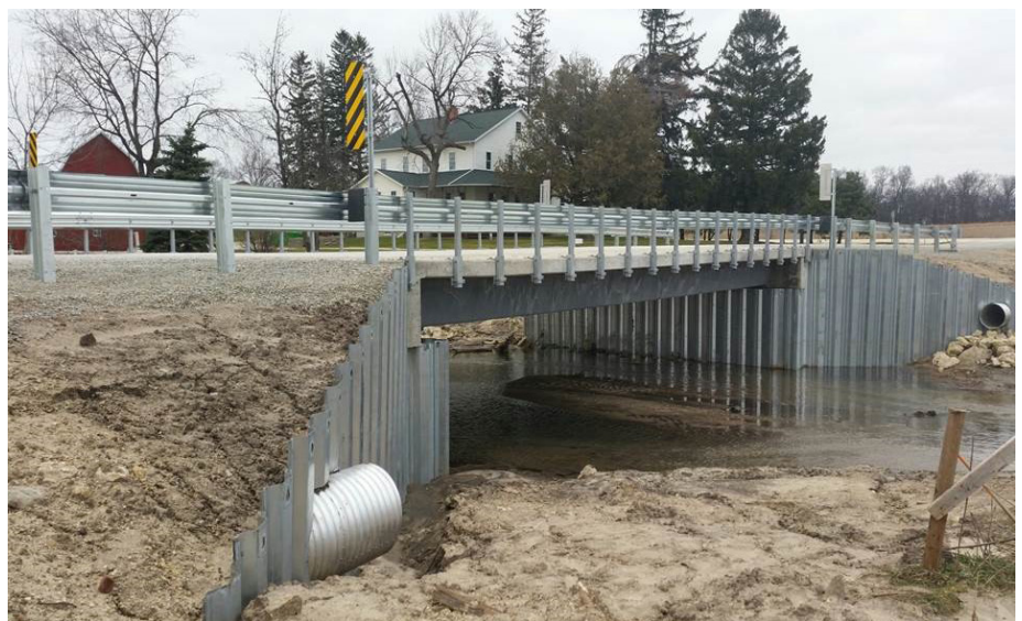
The Amish Sawmill Bridge is a single-span folded plate tub girder bridge with a span length of 52 ft and a roadway width of 30 ft
