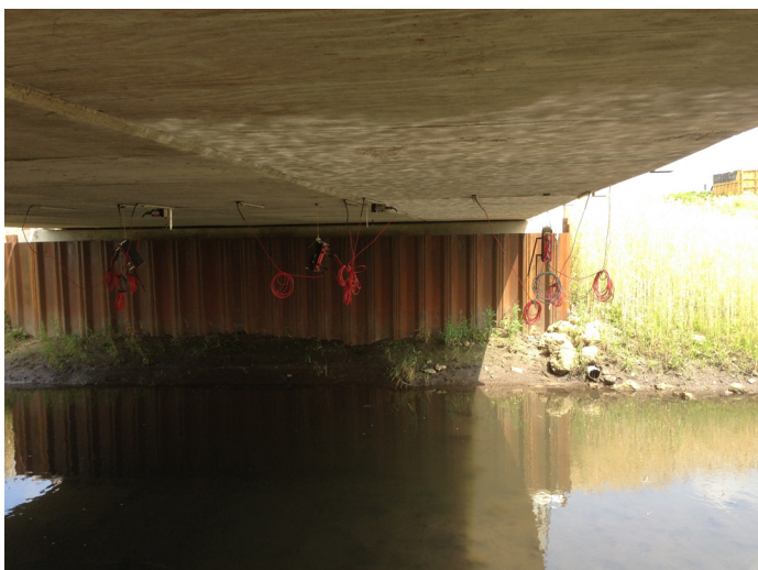
Profile view of completed GRS abutment with sheet pile and underside of bridge instrumented for live load testing
