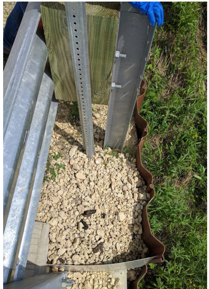
Close-up of completed top fill of GRS abutment with sheet pile outside of bridge rail
