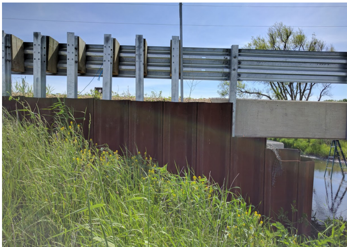
Elevation view of completed GRS abutment with sheet pile at deck connection
