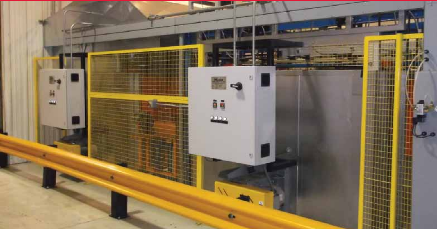
At Left: Photos show the Double HH Manufacturing plastisol oven and dipping process equipment used prior to the installation of the new automated plastisol system. Above: The new automated plastisol system, based on a preliminary design by Iowa State's Mechanical Engineering Capstone Design Program students, was installed at Double HH Manufacturing in the spring of 2012.
