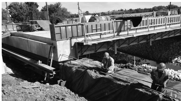
The Iowa DOT constructed a slide-in bridge project on Iowa 92 near Massena, Iowa in 2013. Photo courtesy of the Iowa DOT.
