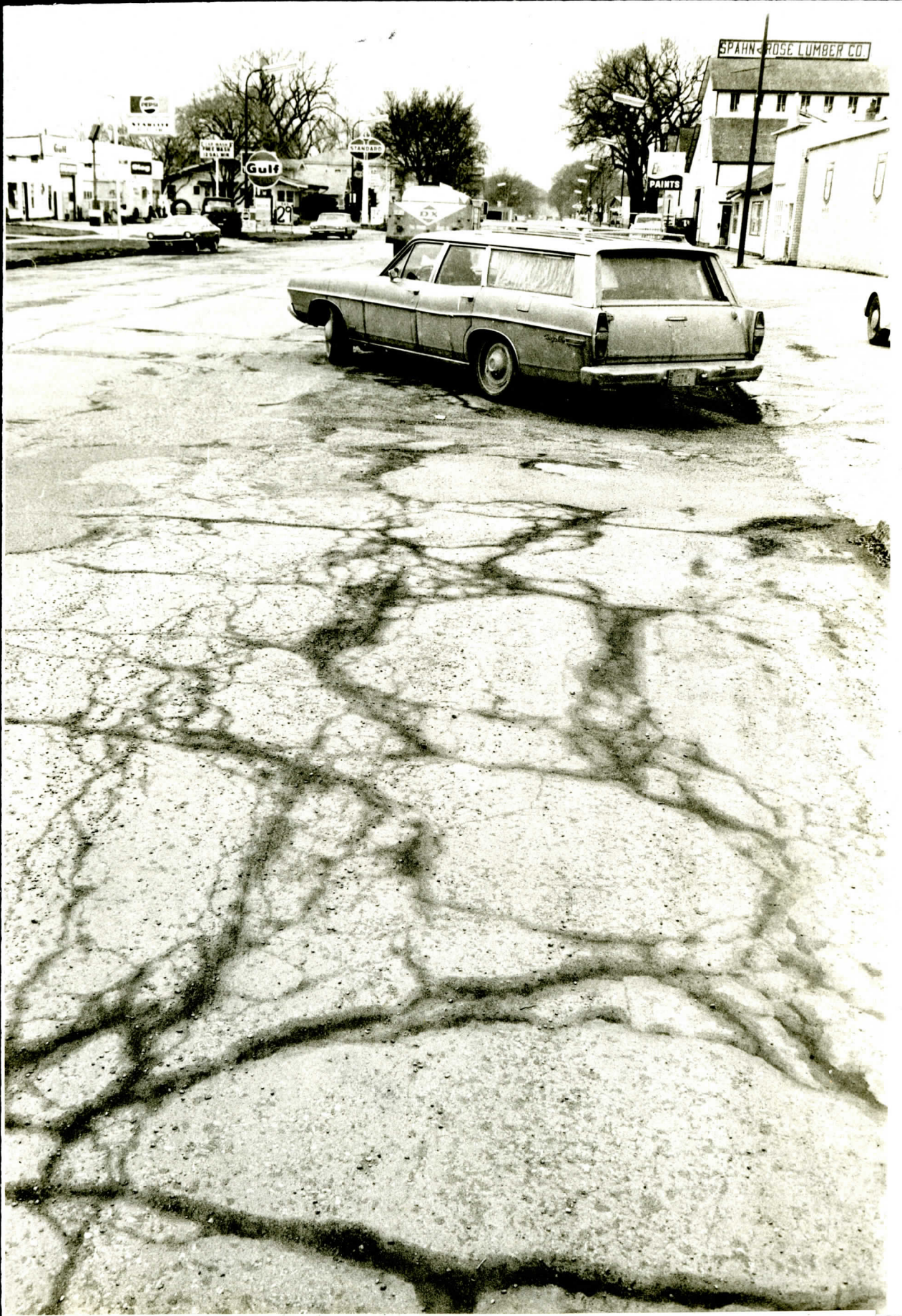
Highway 9 (Main Street, between Fifth and Fourth) - Surface and structural deterioration.
